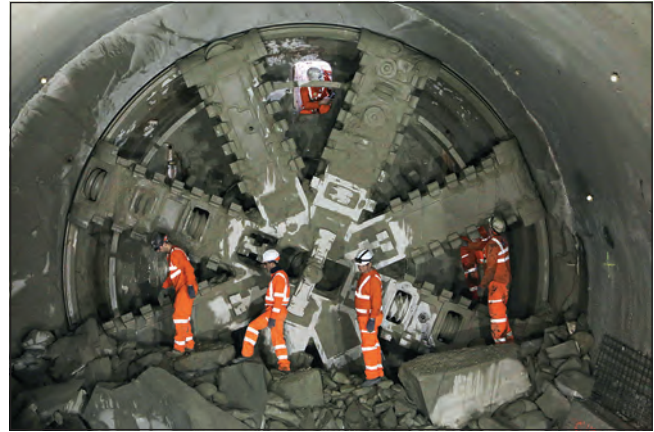
Figure 12. Tunnelling was completed in June 2015, moving the project into a major handover phase
