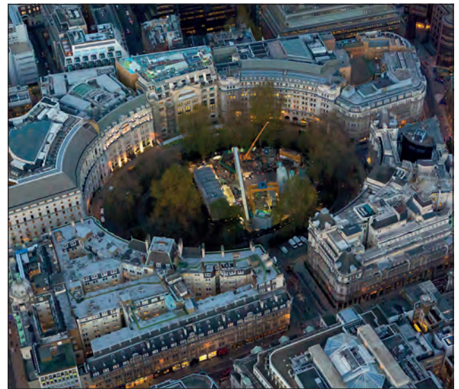
Figure 11. Tunnelling for Liverpool Street station being carried out from Finsbury Circus – detailed procurement strategies were prepared and agreed for all contracts
