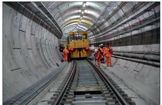
Figure 15. Rail systems installation in the running tunnels is part of the system-wide works
