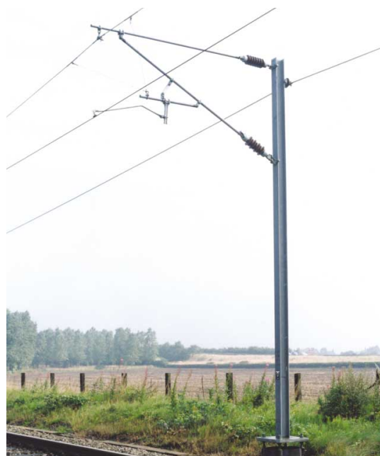
Overhead Electrification Example
