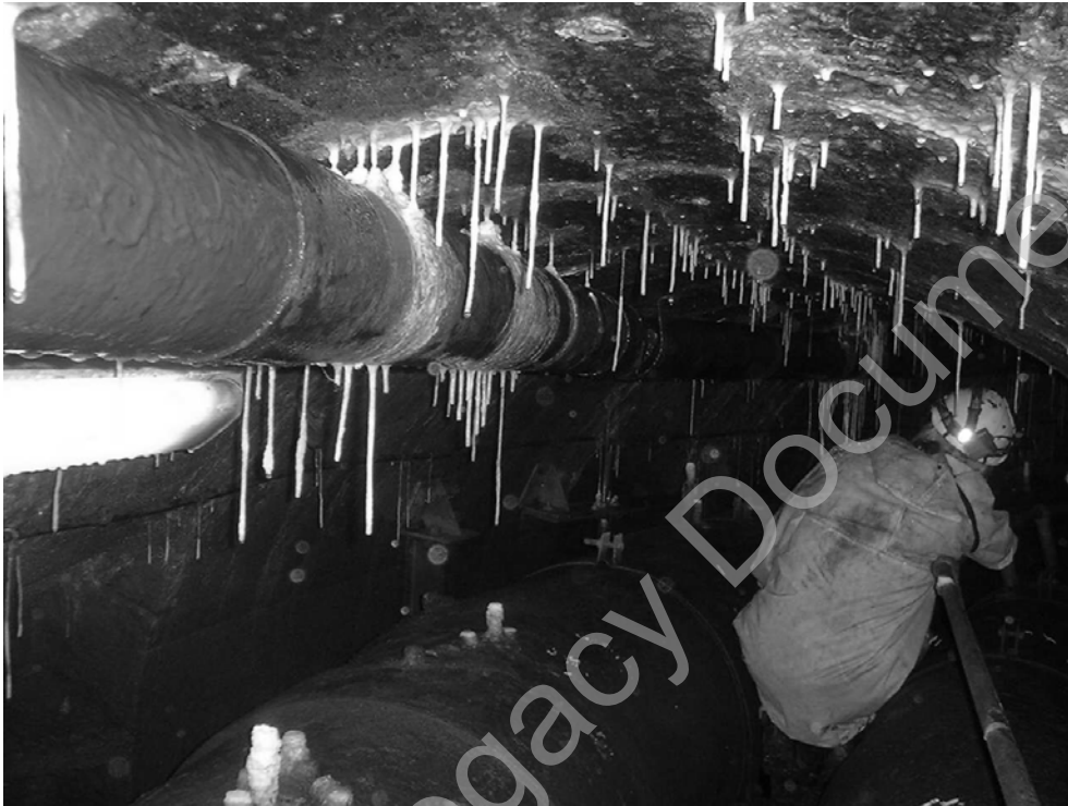
Figure Caption: e.g. Figure 1. Tunnel deterioration
