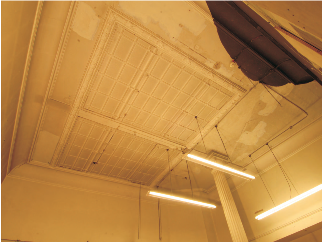
Fig 18 Blocked skylight in rear ground floor of 9–15 Oxford Street
