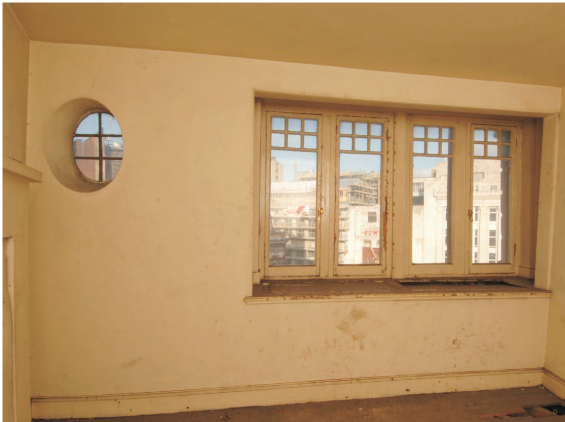
Fig 31 Fourth floor window in 7 Oxford Street showing exposed flaps in window seat
