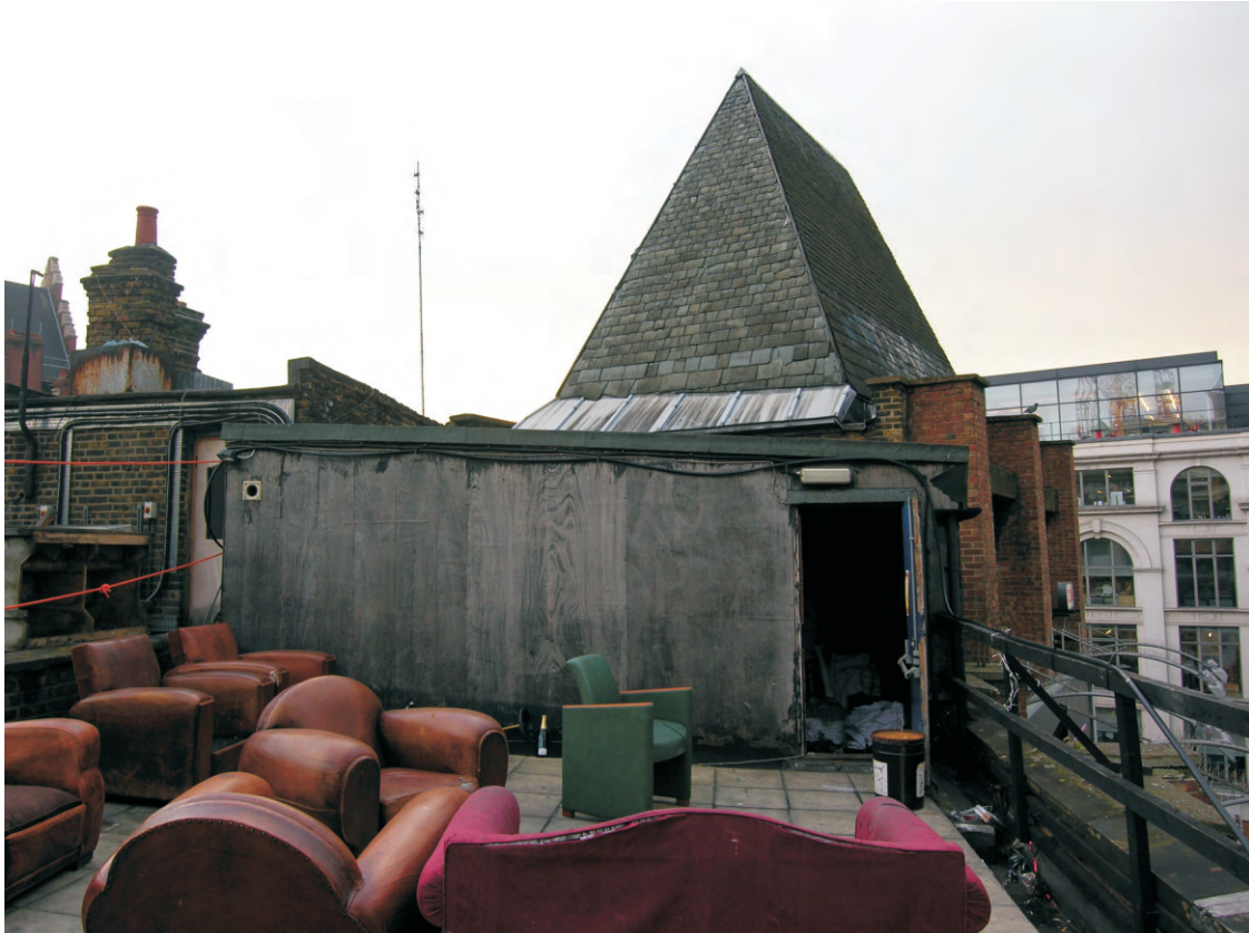
Fig 60 Flat roof of 148 Charing Cross Road, giving access to interior of tiled pavilion roof
