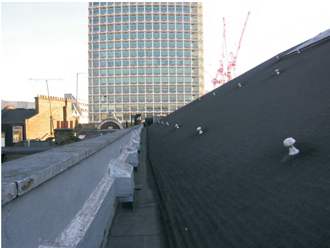
Fig 45 Roof of Astoria showing brick piers at base of parapet around the roof
