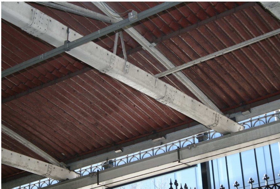
Plate 42: Detail of truss showing trough riveted together with plates of varying widths
