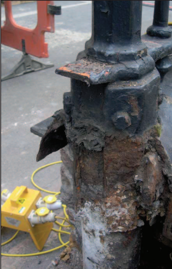
Plate 8: Exposed railing post
