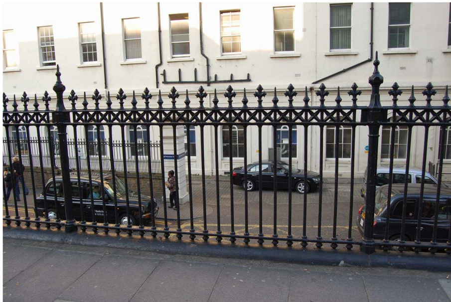
Plate 14: Western section railings, panel 44, metal clamp to centre of high level rail
