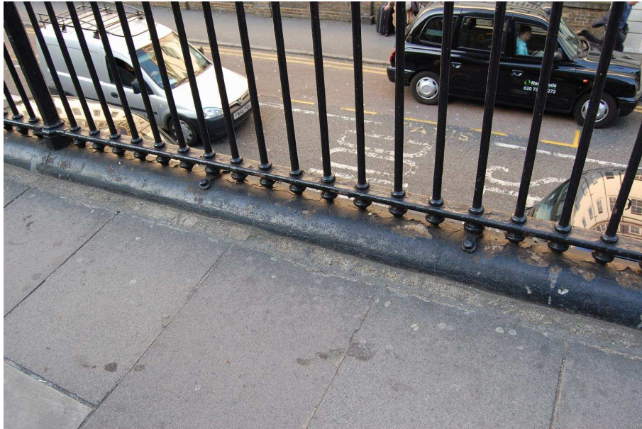
Plate 13: Western section railings, panel 42, balusters bolted to base
