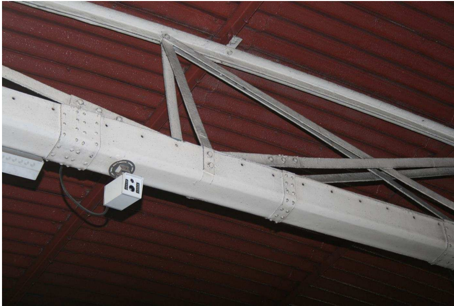
Plate 43: Detail of truss showing struts attached to the outside of the trough
