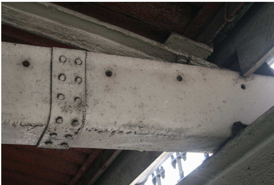
Plate 44: Detail of residual holes to truss
