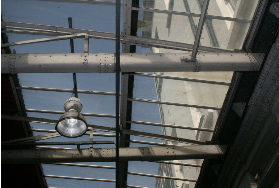
Plate 45: Detail of repair to northern end of a truss (upper) contrasted with the unrepaired truss (lower)
