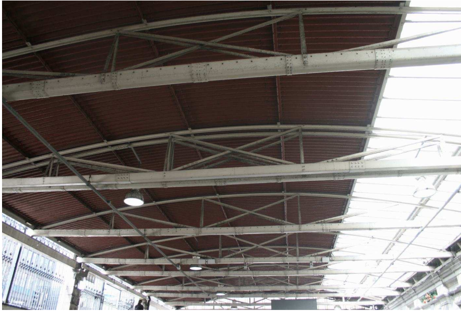
Plate 47: Detail of truss type 2 showing fewer plates and larger rivets in comparison to the type 1 trusses
