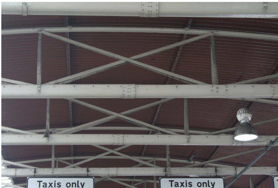
Plate 46: Detail of truss with possible repaired strut running into the interior of the trough
