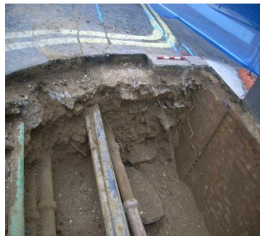
West facing section at east end of trench. Showing pre-existing services and modern brick built retaining wall on right
