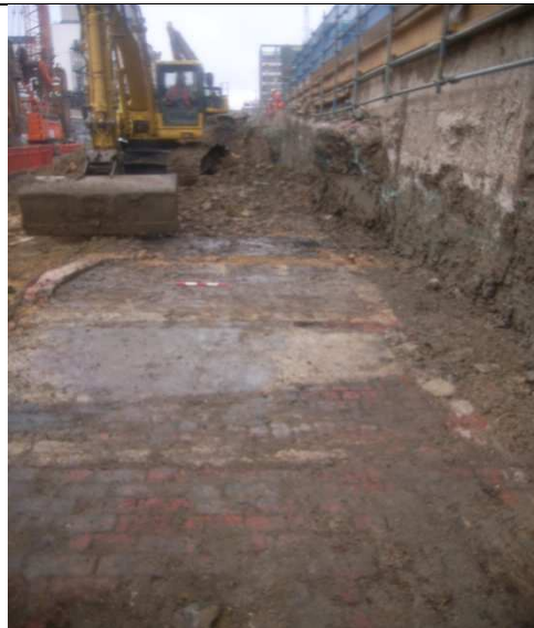
Base of cellars (6546) brick floor (6545). Looking east. The southern diaphragm wall of the Station Box is on the right
