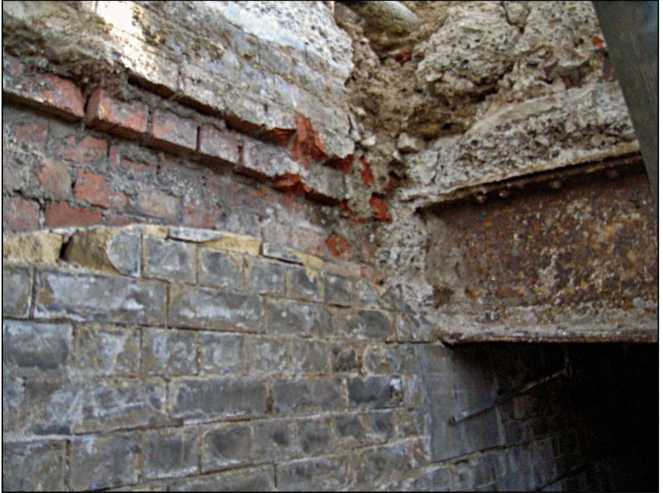
Plate 20: Steel girders within Milk Ramp and northern wall of Ramp. Looking north
