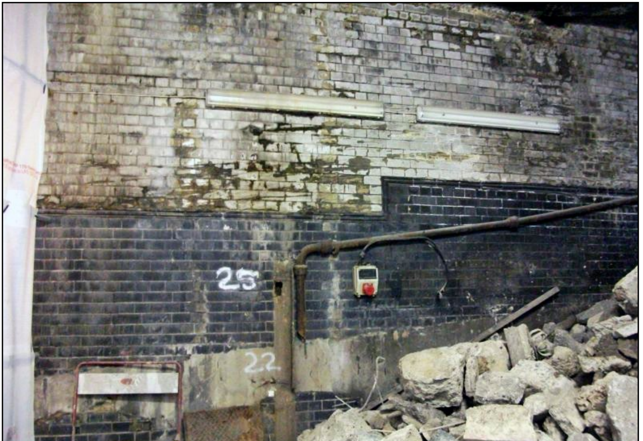
Plate 26: Lower section of Retaining Wall with scars of vehicle impacts
