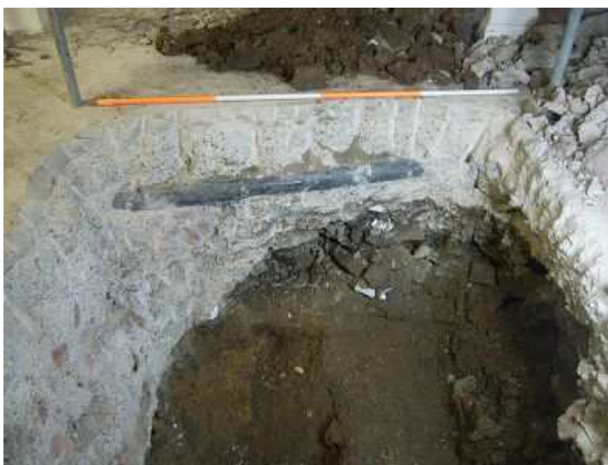
Plate 4: Test Pit 4, Brick-filled void beneath concrete slab
