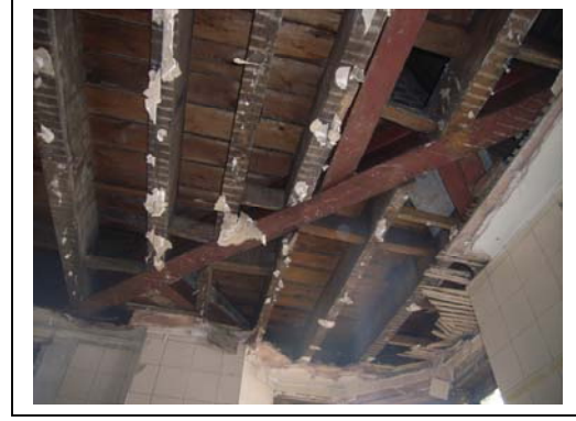
Plate 4: steel joists within floor at north-east corner of 96 Dean St supporting projecting bay
