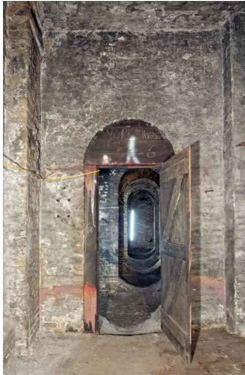
Fig 10 View of the eastern door to the mess room (Room 9) and five storage cabins (Rooms 8, 7, 6, 5 and 4), looking east
