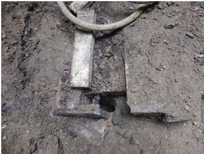
Photo 20: Photo showing the western end of the concrete and brick manhole, looking north
