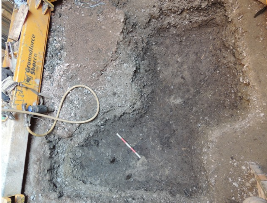
Photo 11: Three stakes from a possible structure pre-dating the Roman road. Twigs from the road foundation can just be seen to the right; looking east
