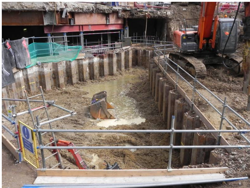
Photo 1, OSD foundation trench, after removal of 0.5m of piling mat, at 108.90m ATD looking north.
