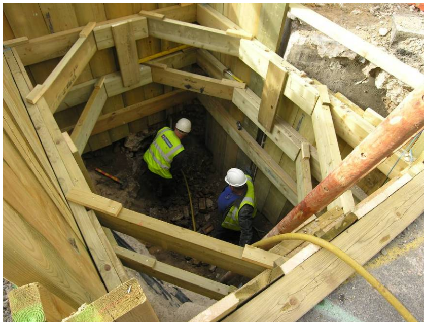
Photo 3 Western Access shaft, removing 19/20th-century building foundations and north–south aligned wall [20], looking south-east
