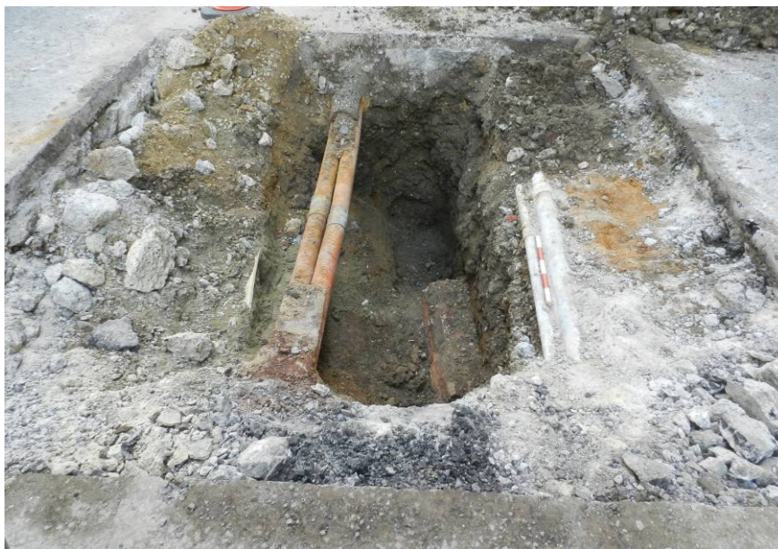
Photo 2 Trench A with intercutting gas pipe and telecommunication duct trenches beneath the concrete, backfilled with sand, gravel or re-deposited soil [2], sealing a truncated c 18th to 19th-century red brick wall [3]. Looking east.
