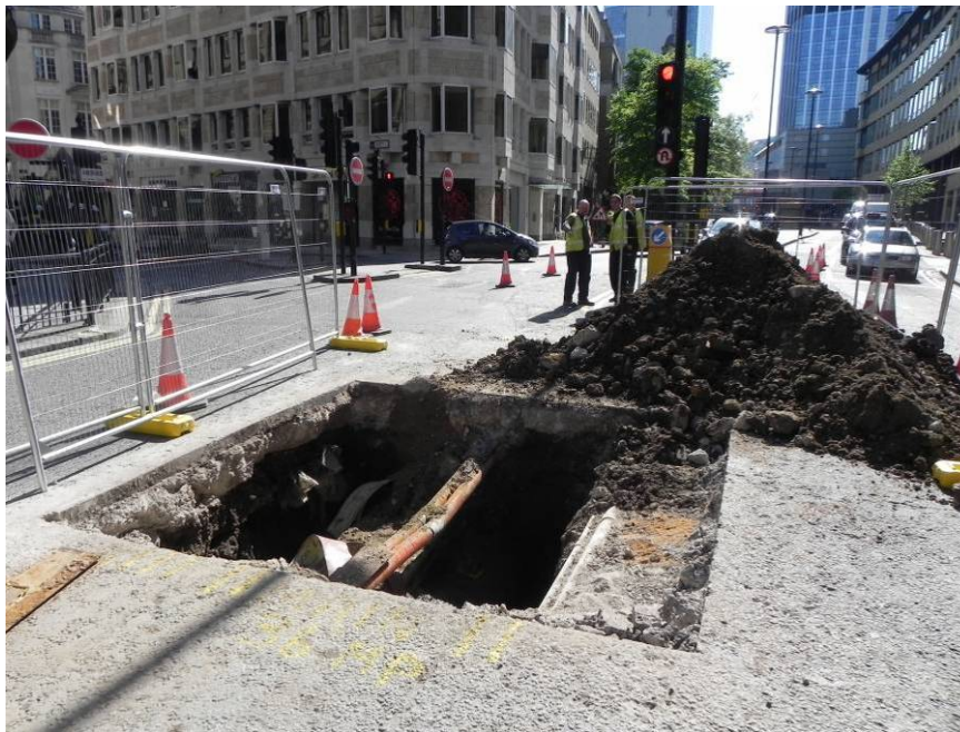
Photo 1 Location of Trench A at the junction of Blomfield Street (top left), looking north-east.
