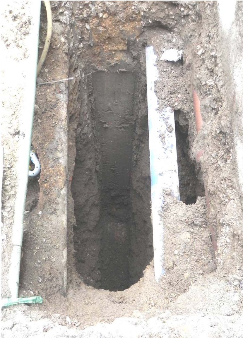
Photo 4 Machine dug sondage within Trench 1, showing a red brick floor at 3.90m bGL. Note: the trench was inaccessible and a closer examination and record of this feature was not possible at this time. East at top.
