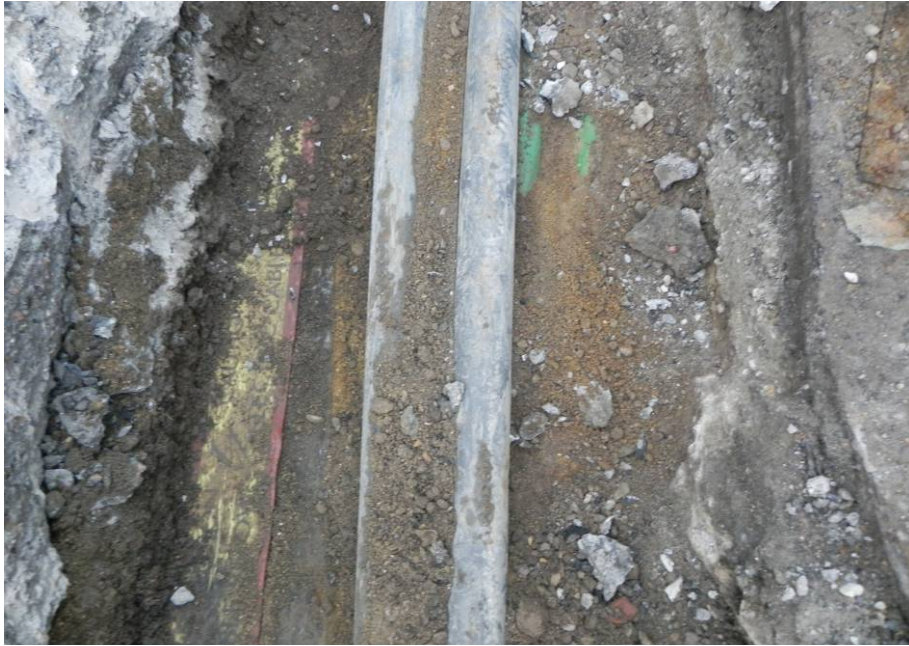
Photo 4: Close up of utilities within the southern half of the trench, with tarmac above concrete left and right. From above, north at top.
