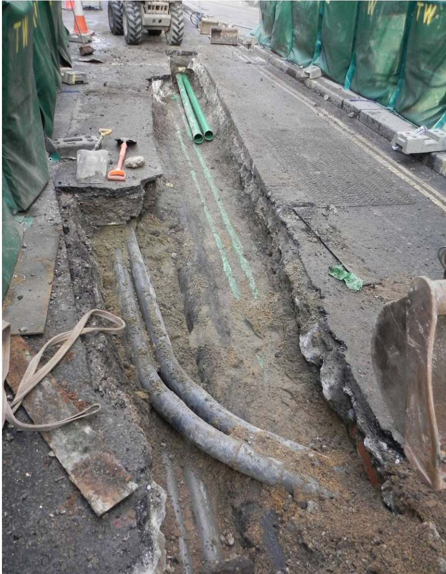
Photo 2: The northern half of the trench, with intercutting gas pipe and telecommunication duct trenches beneath the concrete, backfilled with sand and gravel, looking north-east.
