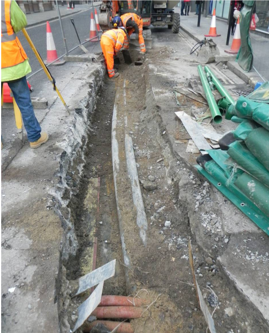
Photo 3: The southern half of the trench, with intercutting duct trenches beneath the concrete, backfilled with sand and gravel, looking north.
