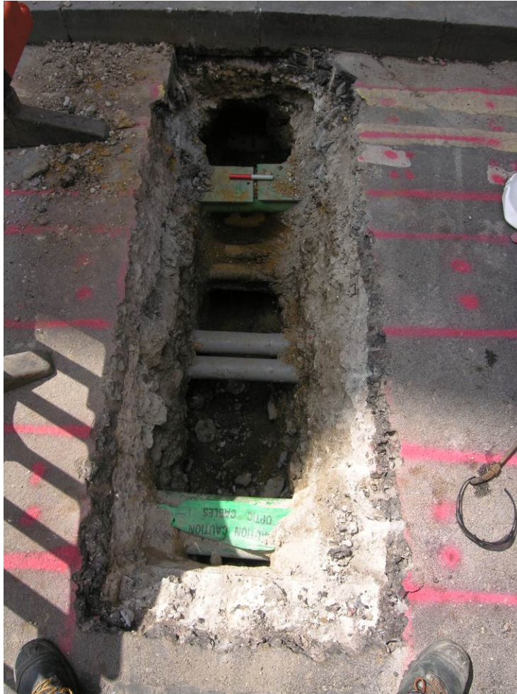
Photo 3 Trial trench TM01F, modern services aligned east–west, only modern backfill of utility trenches was exposed, looking north
