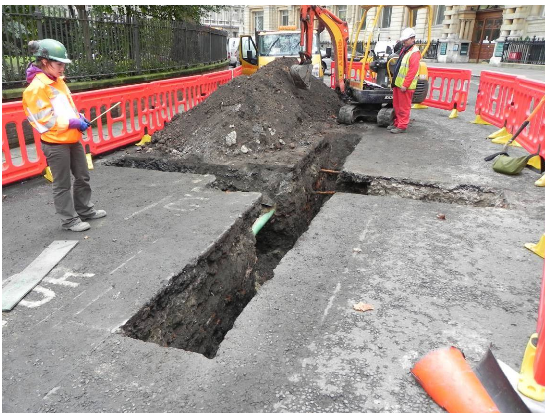
Photo 1: Western grout shaft trial trench. Telecommunications services (green cable) visible at centre. Facing south.
