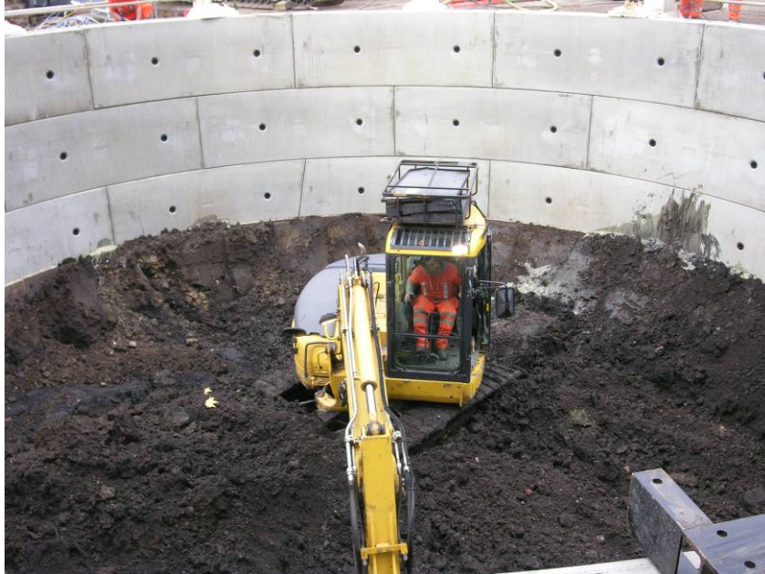
Photo 2, general watching brief, machine excavating post-medieval dumps at 3m below ground level, looking south.
