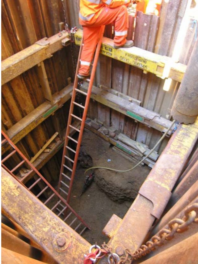
Photo 1 RBS trial trench looking north. Natural sandy gravels exposed between 2.9 and 4m bGL
