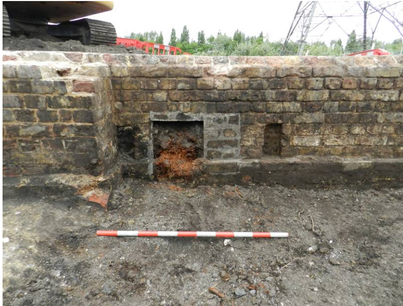
Photo 3 Recess for a possible floor. A portion of rotten timber remains in situ. (Looking north east)
