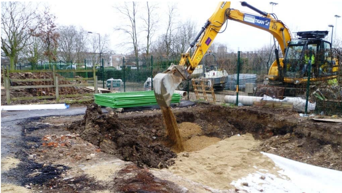
Photo 24 Sand filling trench 3 to 200mm above brick remains at side of wall [47]
