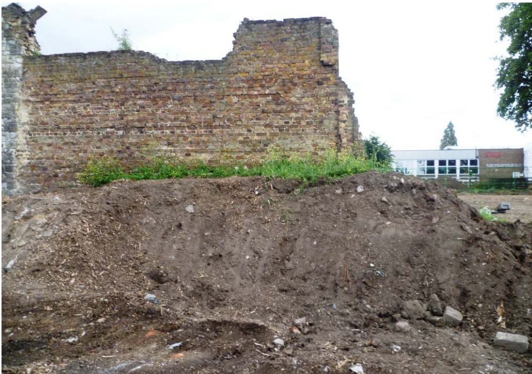
Photo 8: Ground reduction north of the freestanding Congregational Church wall (first metre removed, looking south)
