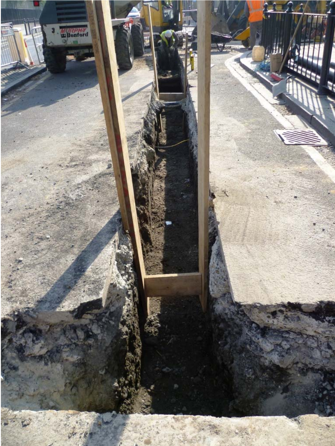
Photo 14: Cable trench looking east along Stepney Green Road
