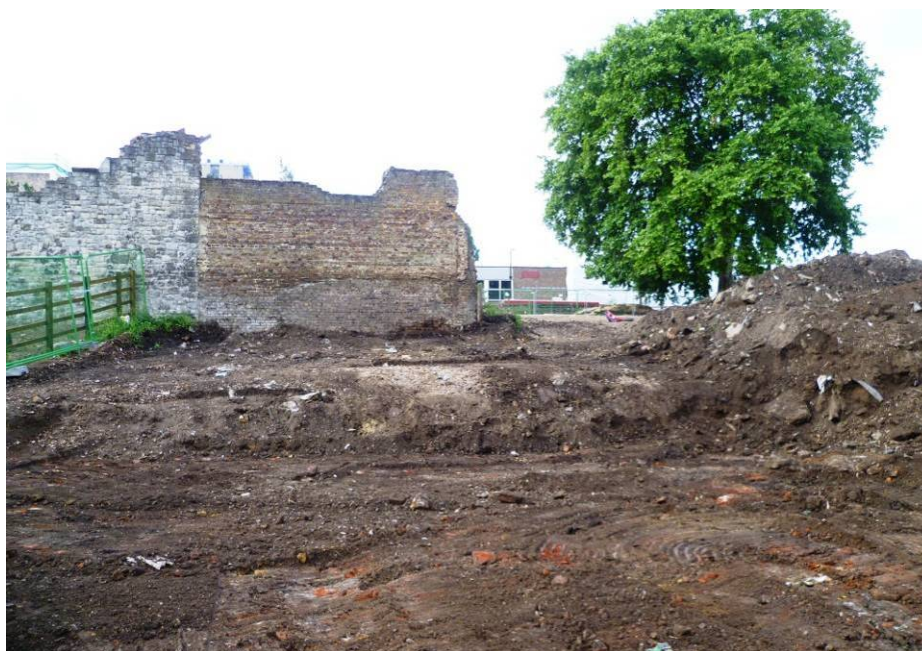
Photo 9: Ground reduction north of the freestanding Congregational Church wall (second metre removed, looking south)
