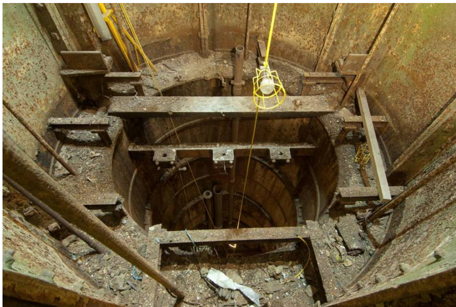
Fig 12 Remnant equipment at the bottom of the upper part of the well (08512027)
