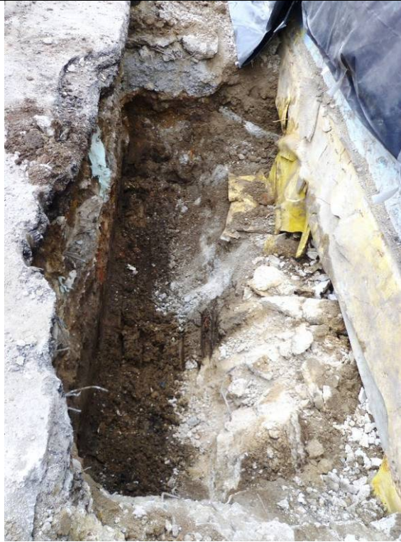
Photo 4: Canopy foundation, third stanchion from west of the southern row (left, looking east), dug into archaeologically sterile natural brickearth and gravel
