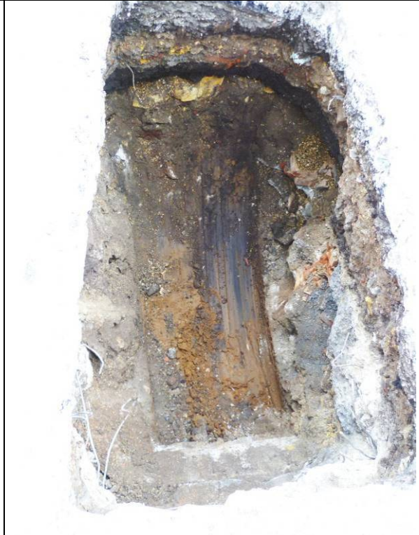
Photo 5: Canopy foundation, stanchion furthest east of the northern row (right, looking west): showing Albion Brewery Concrete foundations cutting through post-medieval coal-ashy nightsoil quarry fills, dug into archaeologically sterile natural brickearth and gravel
