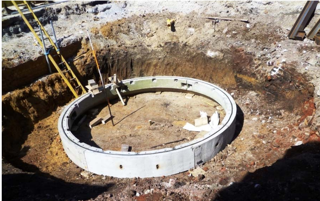
Photo 7: Thames Water Storm Relief Sewer Shaft: Looking north-west, showing clean natural brickearth at the base of the shaft, darker filled feature to the right of the ladder, red-brown soil, cut through by a quarry and a 19th-century culvert
