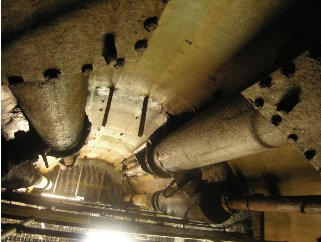
Fig 13 Hydraulic pumping machinery within the shaft below the pump house.
