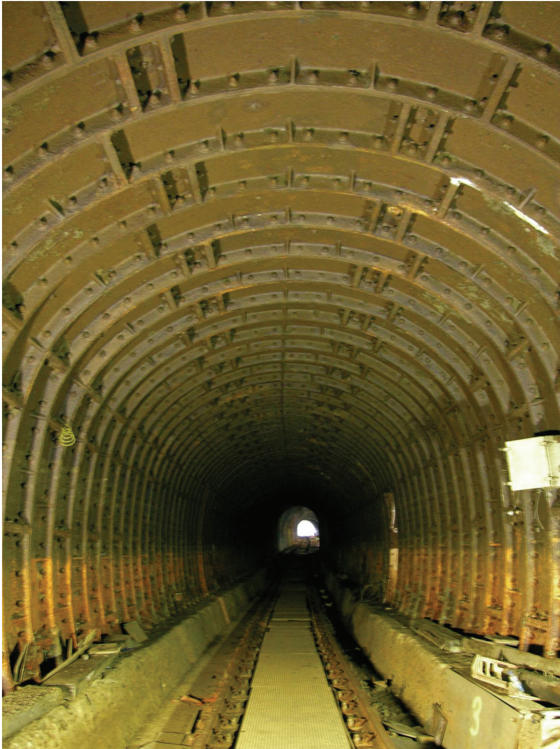
Fig 7 View of the iron-banding incorporated to the central sections of the twin tunnels during works to lower the depth of the Albert Dock in 1935, looking south.
