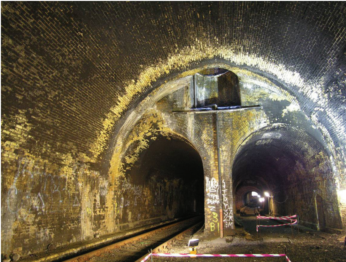
Fig 6 View of the transition between single tunnel to twin tunnels with an air vent above , looking south.
