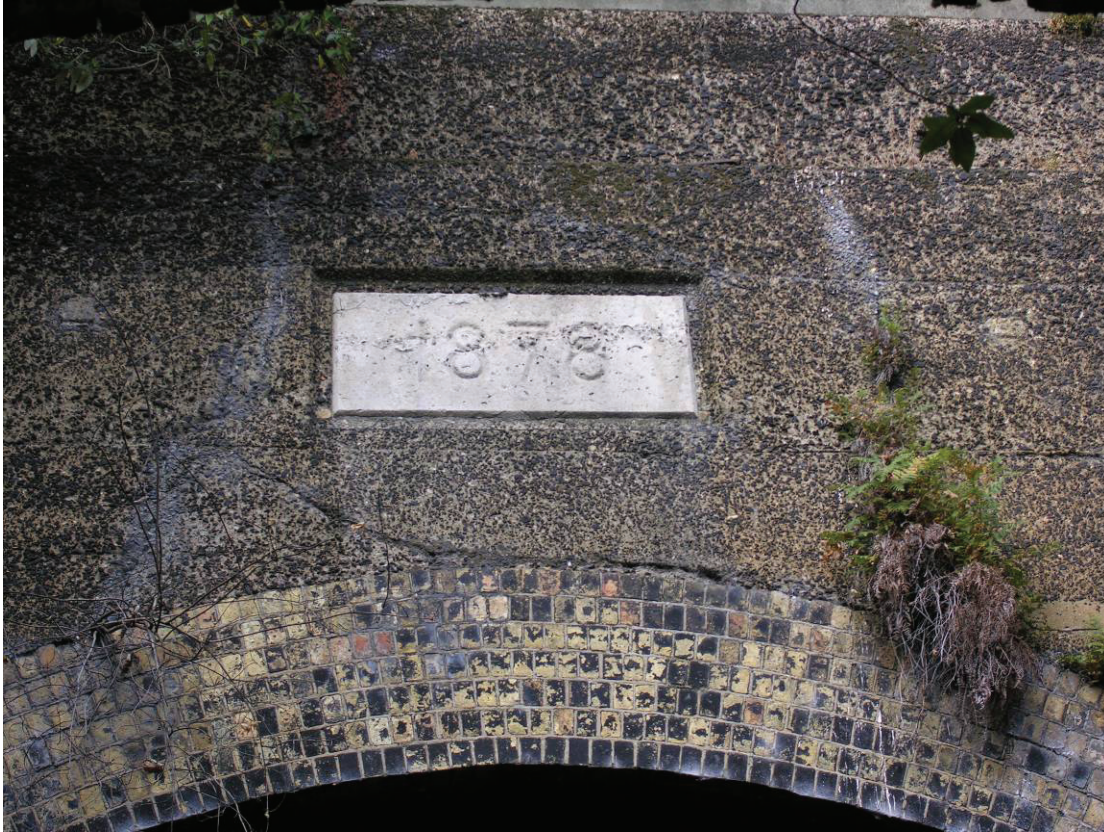
Fig 4 A view of the stone date panel above the tunnel portal, looking north.
