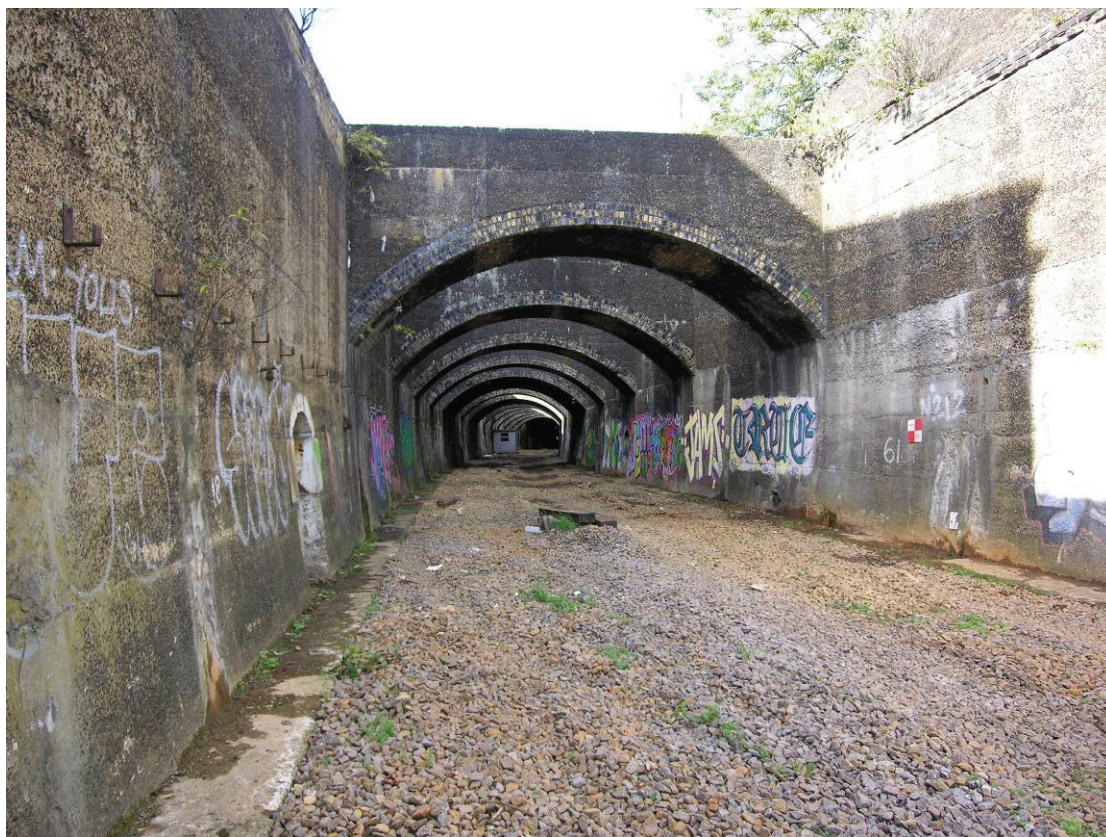
Fig 2 A general view of the 19th century concrete-lined cutting and flying buttresses leading to the tunnel portal, looking north.
