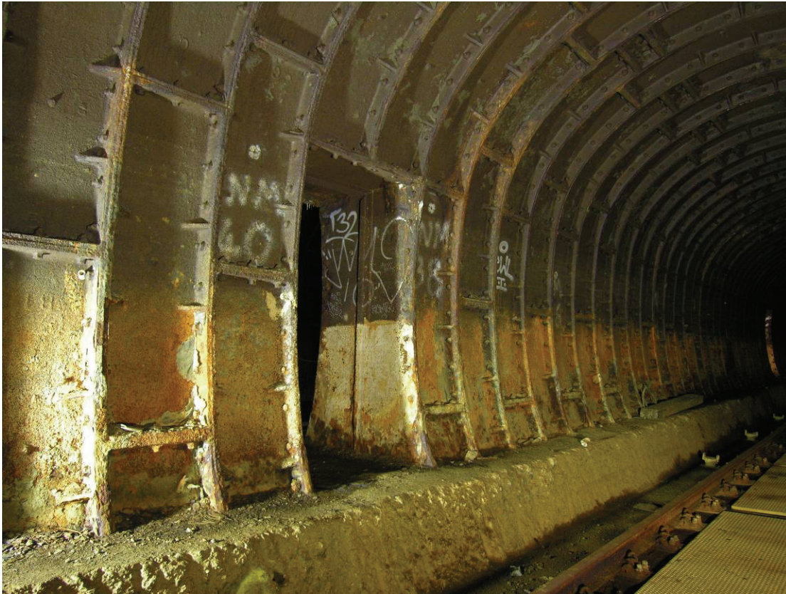
Fig 8 Detail of the iron banding with an opening linking the twin tunnels, looking south-east.
