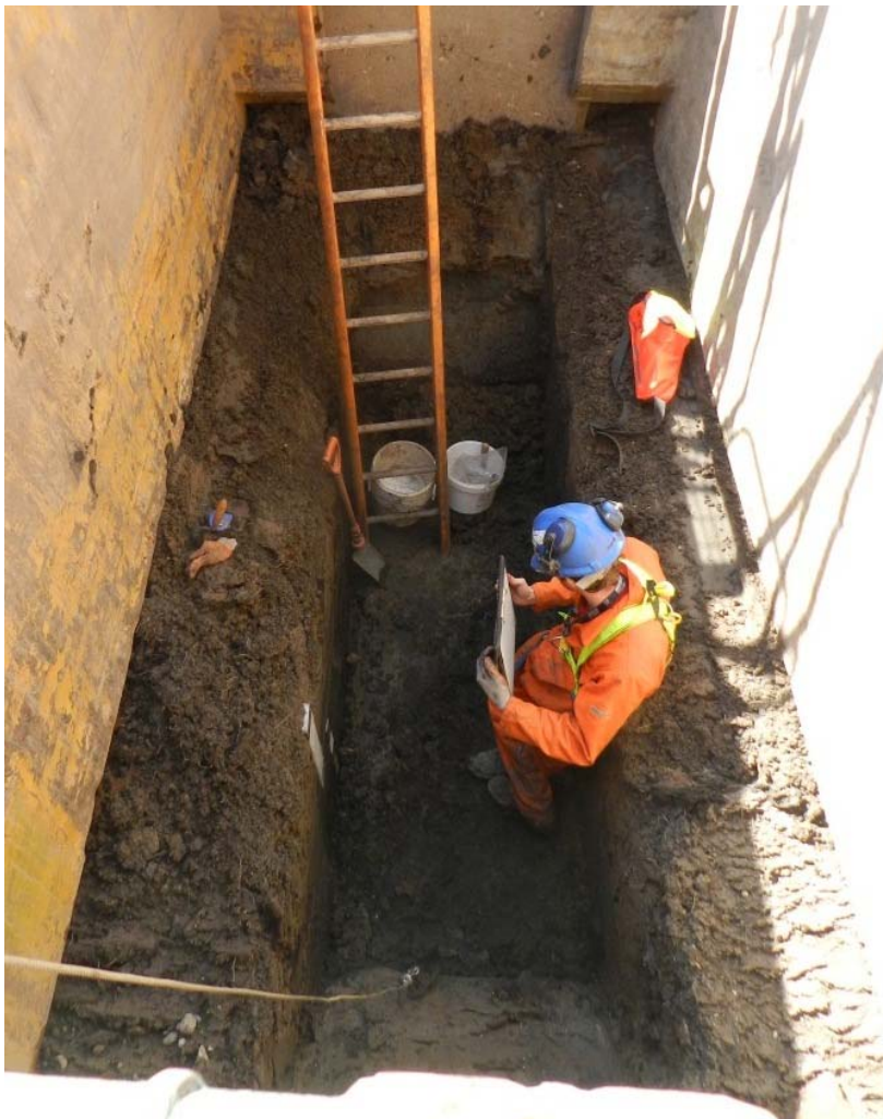
Trench 4: sampling the base of alluvial clay and top of wood peat
