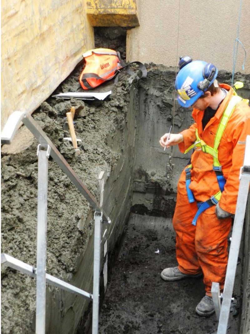
Trench 3: sampling the base of the upper alluvial clay and top of wood peat
