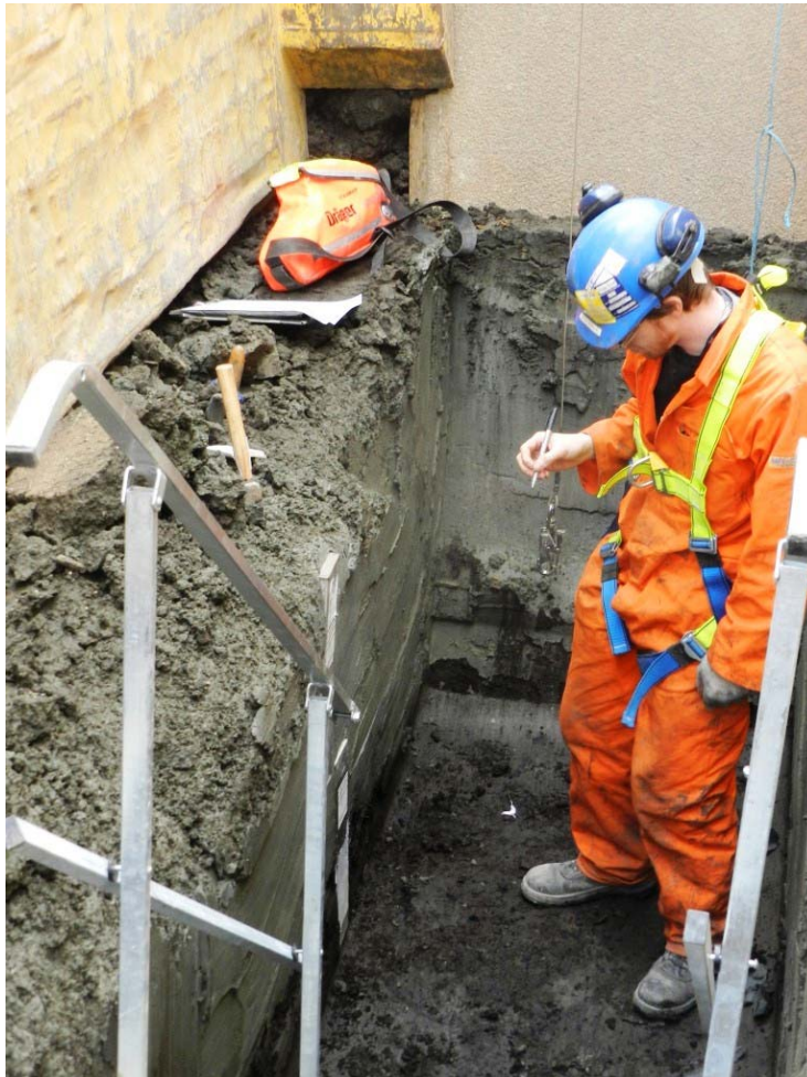
Photo 5 Trench 3: sampling the base of the upper alluvial clay and top of wood peat
