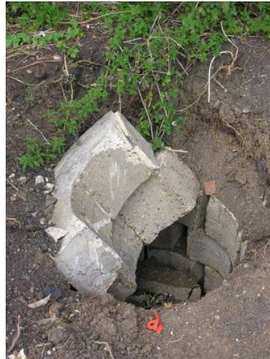
Fig 14 The remains of the air vent to the west of the shelter
