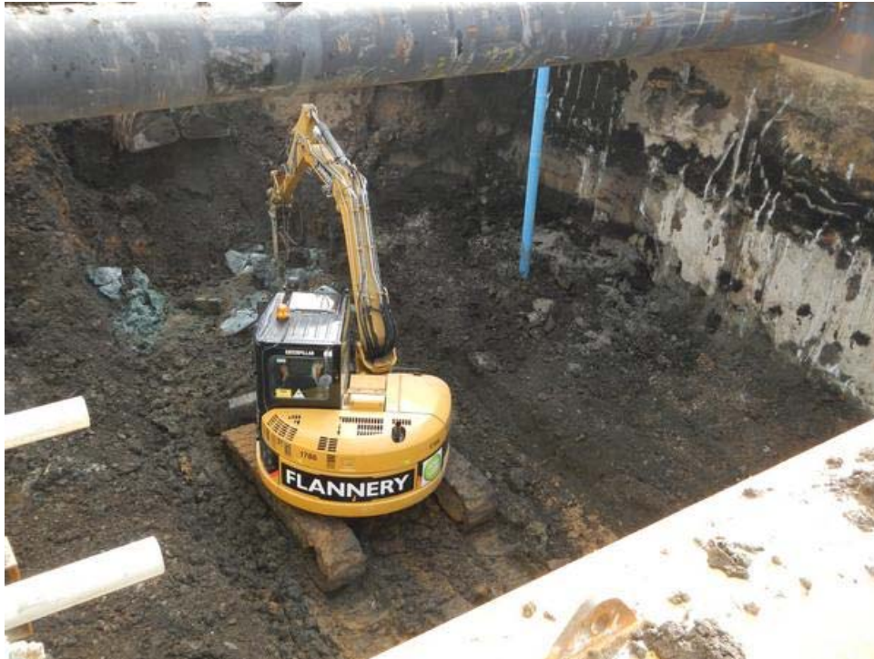
Photo 15 View through the deposits during ground reduction at the east end of the site (looking southeast)
