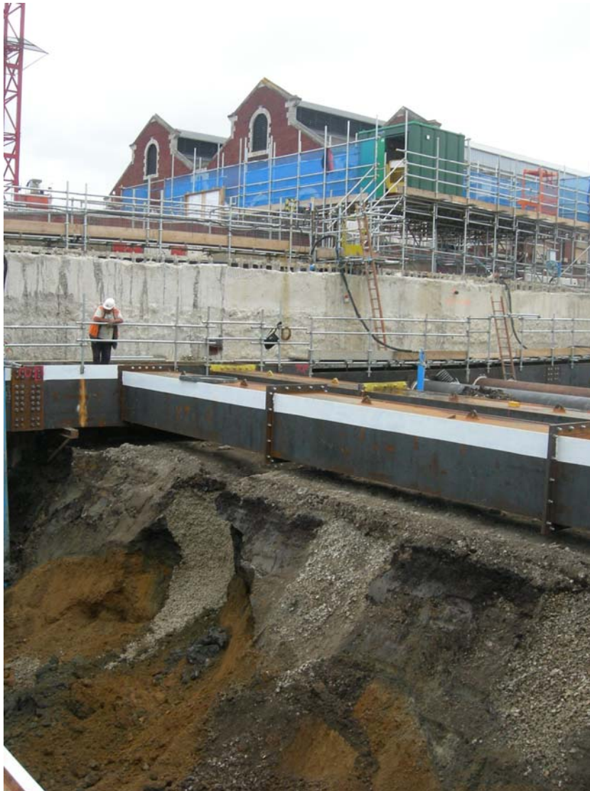
Photo 14 View through the deposits during ground reduction at the west end of the site (looking north east)
