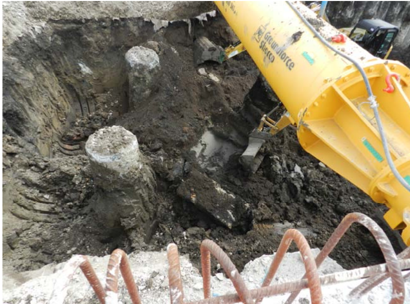
Photo 16 View through the deposits during ground reduction at the eastern end of the site in the Marmadon Sewer (looking south)
