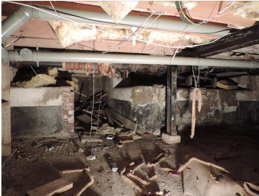
Fig 18 The Phase 1 cellar, looking east. Note the stillages and blocked cellar drop between them.
