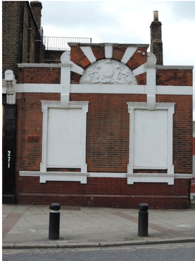
Fig 13 East elevation of the north end block of the building, looking west
