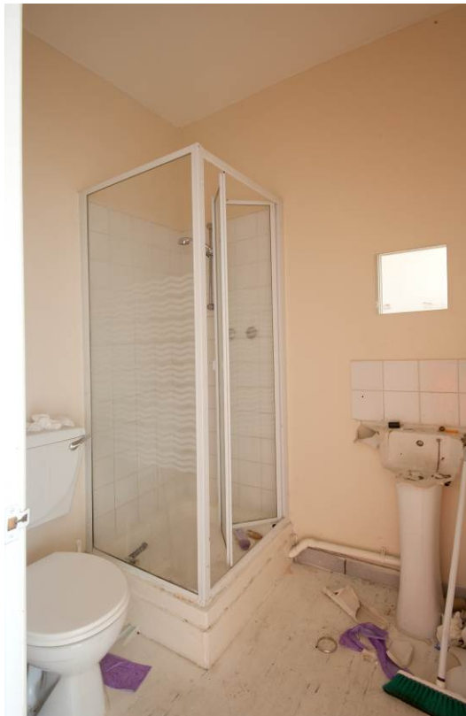
Fig 23 Representative first floor en suite bathroom from a single occupancy hostel bedroom
