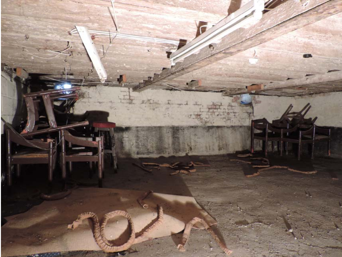
Fig 5 View of part of the cellar beneath the early 20th century extension, looking north
