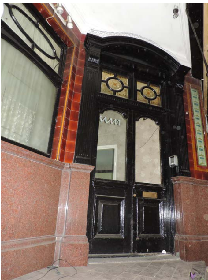
Fig 2 A view of the entrance lobby on the east elevation, looking north-west
