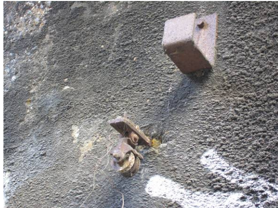
Photo 46 A pulley wheel and cable bracket on the south-western site of the southern cutting
