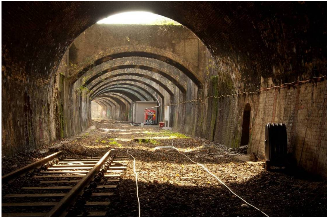
Photo 41 The view south through the southern portal towards the buttresses of the southern cutting.
