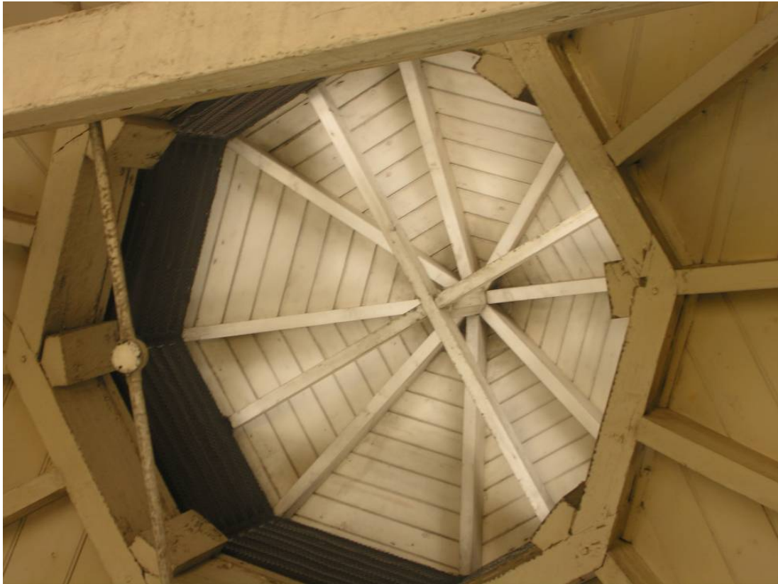
Photo 11. Detail of the interior of the louver in the pumphouse roof, with the king post resting on the two small cross beams.
