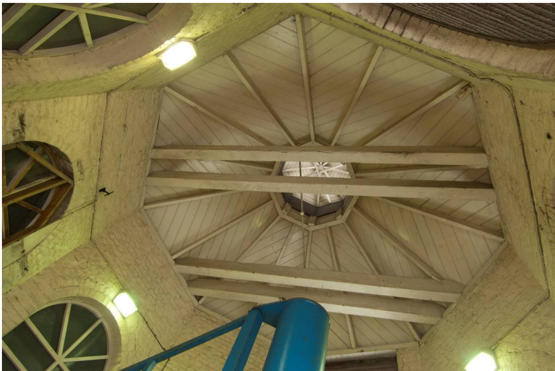
Photo 10. The interior of the roof of the pumphouse, looking up and to the north.
