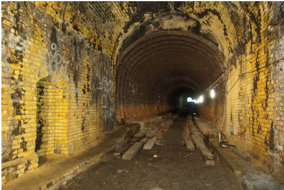
Photo 34. The southern end of the western brick twin tunnel, looking south east towards the steel twin section with a refuge on the left.
