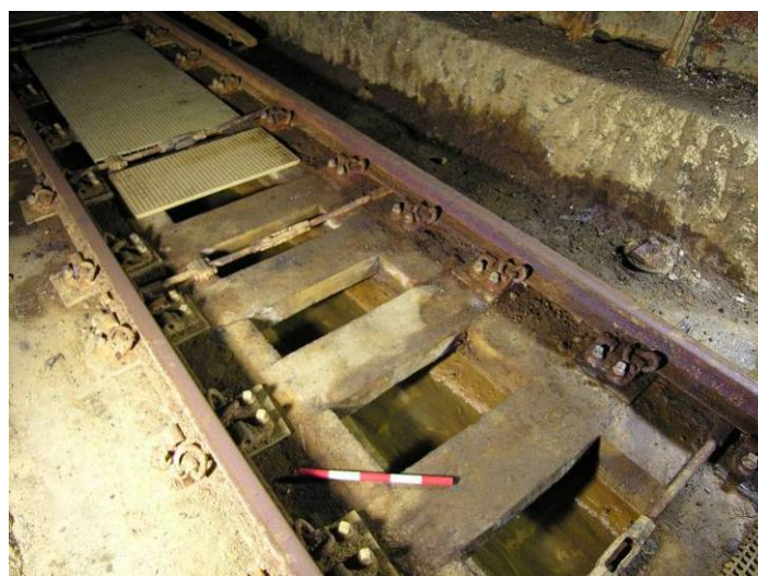
Photo 37. The open culvert running beneath the sleepers in the steel lined section of the tunnel.
