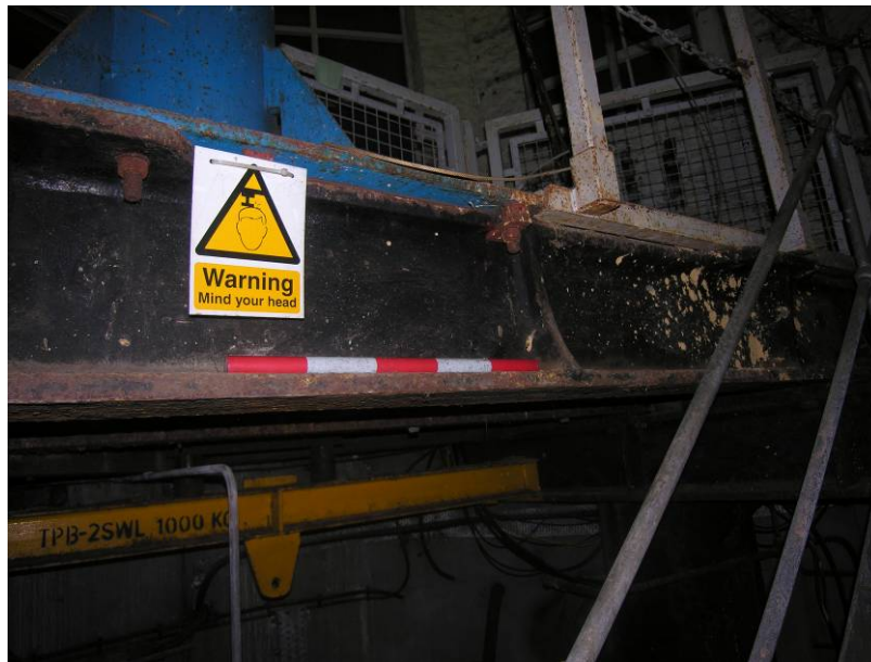
Photo 16. The possible 19th century wrought iron joist across the centre of the shaft opening, used to support the modern hoist.
