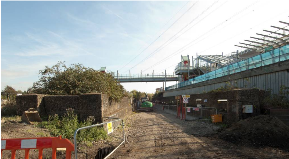
Photo 22. The northern entrance to the cutting of the Connaught Tunnel looking east.
