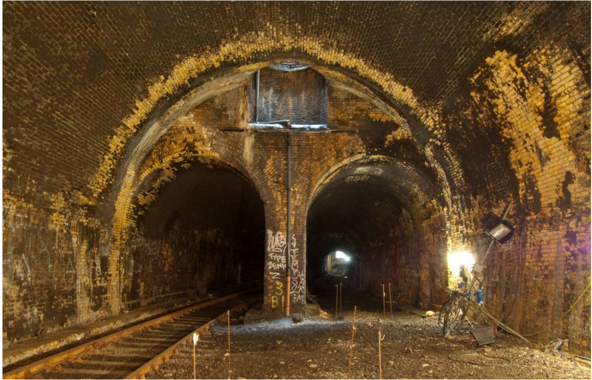
Photo 30. The junction between the north single tunnel and the north twin tunnel sections, with the base of air shaft, looking south east.
