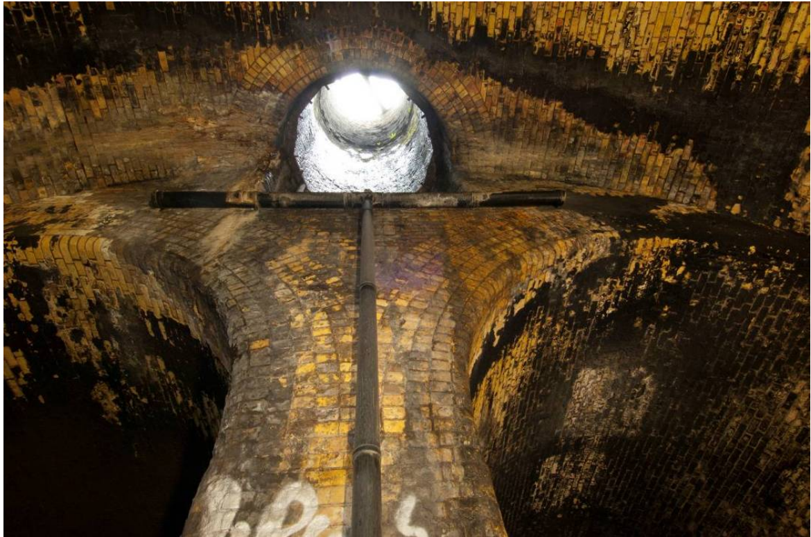
Photo 31. The view up and to the south east at the north [portals of the twin tunnels showing the base of the northern air shaft.
