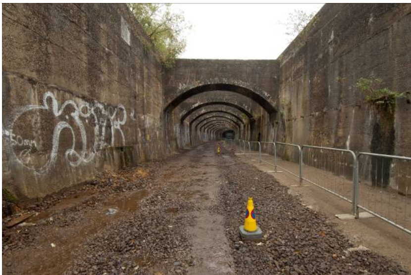
Photo 1. The cutting and buttresses of the northern approach to the Connaught Tunnel, looking east
