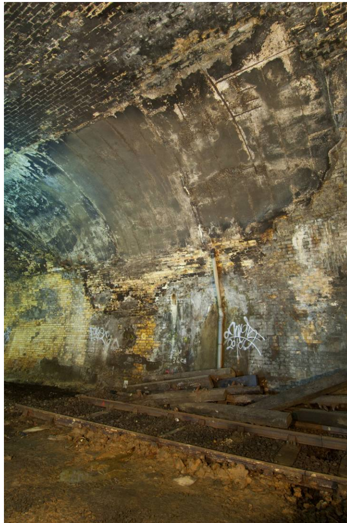
Photo 28. The area of bomb damage repair in the northern single tunnel section, looking north west. Note the reinforcing bars on the right within the concrete and the inserted drain pipe.
