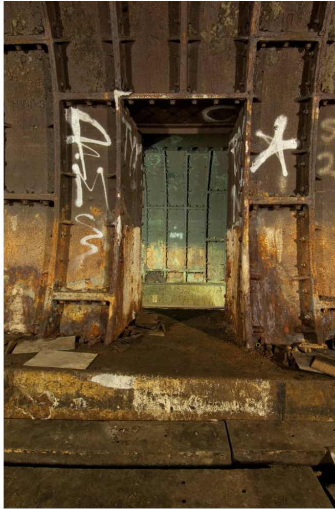
Photo 36 the northernmost of the two cross passages in the steel lined section of the tunnel, looking north east.
