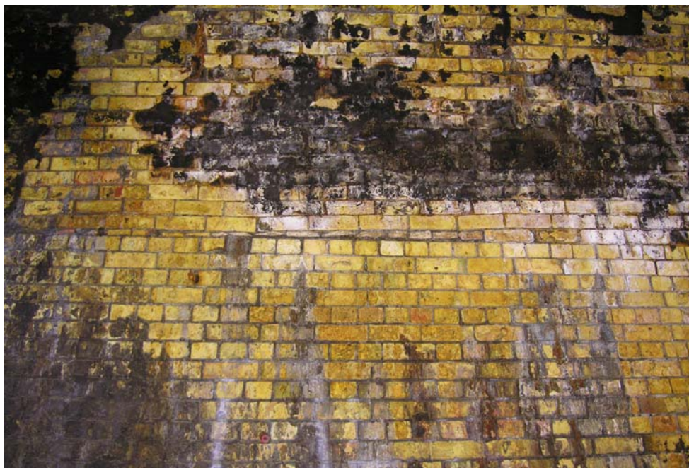
Photo 29. The change in brick bonding from English to stretcher in the northern single tunnel section and the gradual insertion of an extra course of stretcher bricks from left to right.
