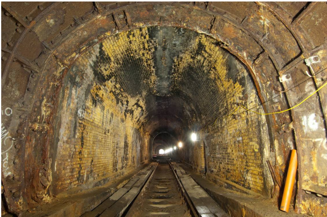
Photo 38 The junction between the steel lined twin tunnel and the southern brick twin section, looking south.
