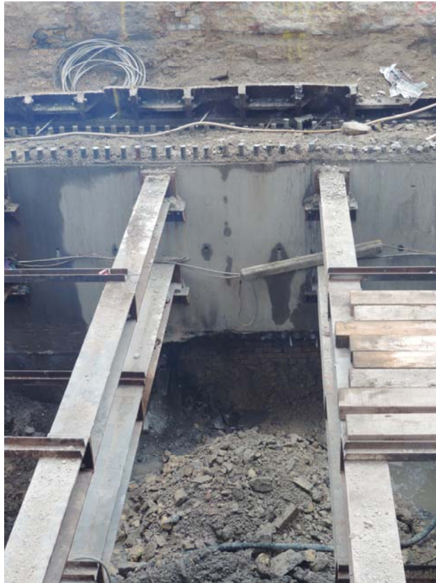
Photo 54 Concrete wall of the new tunnel masking brickwork and steel rings of the former structure
