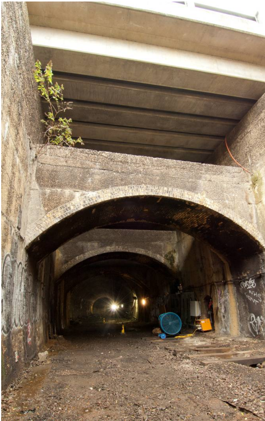
Photo 26 The view east towards the approach to the north portal of the tunnel covered by the concrete structure of the modern road.
