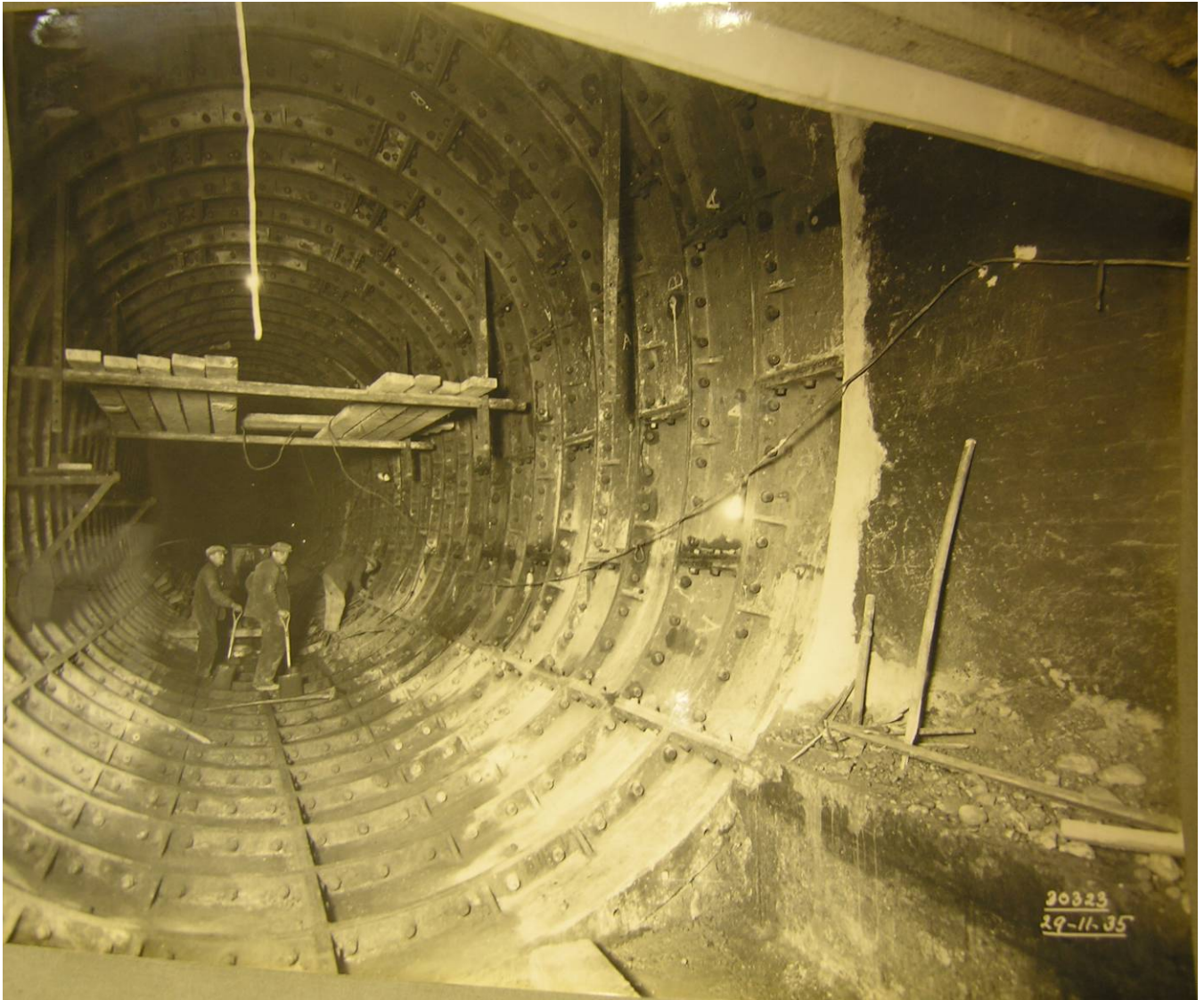
Fig 6. A photograph taken in 1935 during the lowering of the tunnel height and construction of the cast steel central section of the tunnel. (MLDSSC 23896 – Album B)
