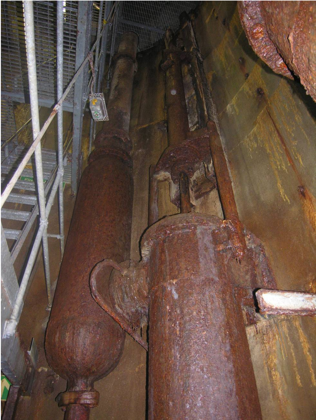
Photo 19. The view looking up and to the south east at one of the two hydraulic pistons and its connection to the extractor pipe which continues up to the top of the shaft and out to the south.
