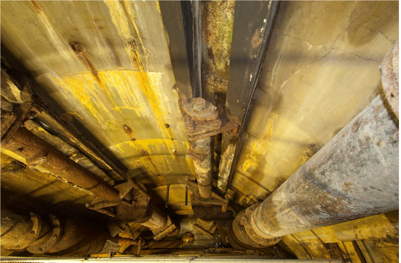
Photo 18. The original pumping mechanism of 1878 on the southern side of the shaft, looking down and to the south. The westernmost of the two hydraulic pistons is in the centre of the photo, the other is on the left.
