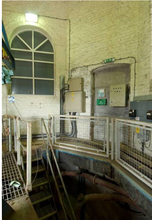
Photo 14. The interior of the pumphouse looking north west, with the steps into the shaft and the blocked doorway in the north elevation.
