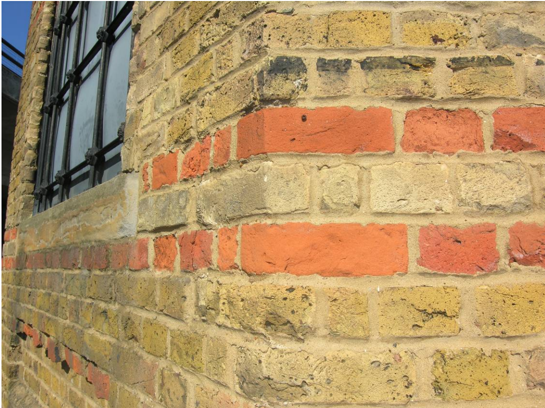
Photo 6. The south west corner of the building looking north showing the three main brick types used in the building's construction, note the King closer bricks on the corner.
