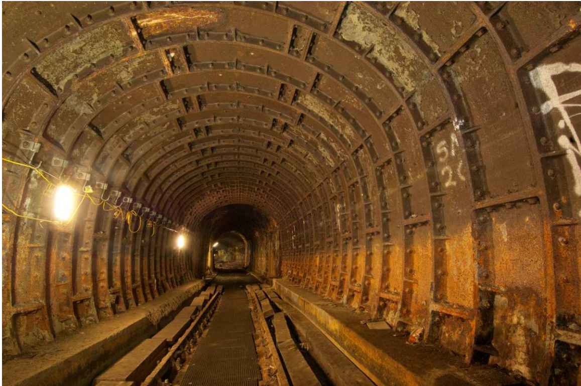
Photo 35 the view north west along the western section of steel lined twin tunnel.
