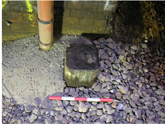
Photo 33. The timber in the track bed between the north portals of the twin tunnel.
