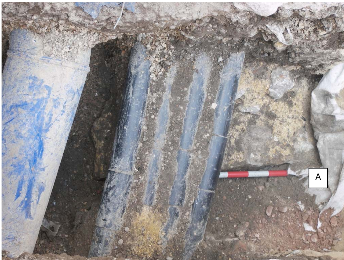
Fig 10 City wall in LIV26, looking north. Wall context [6], earlier exposed in LIV16, continues beneath ducts. Position "A" is the same in both photographs.
