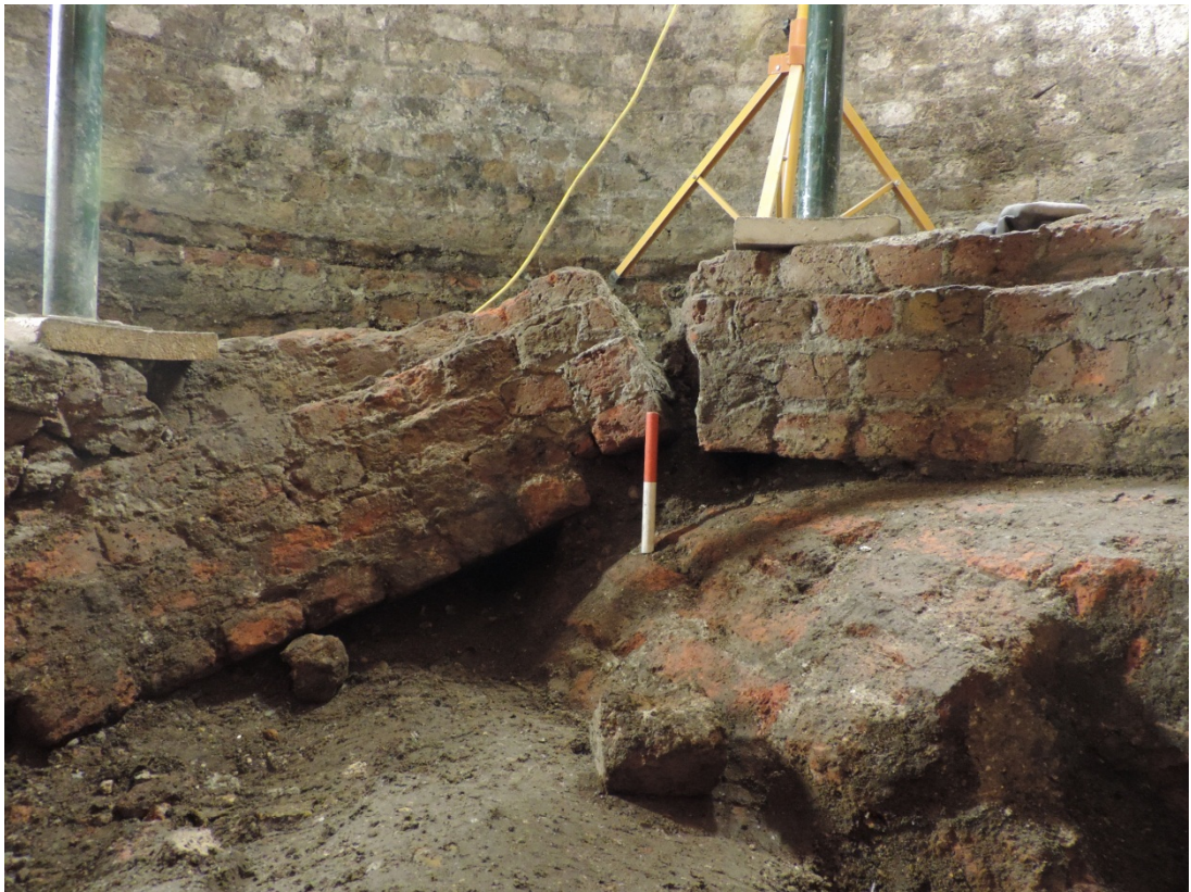
Fig 16 circular brick wall constructed on the 1772 sewer, west side of the wall collapsed (looking south)
