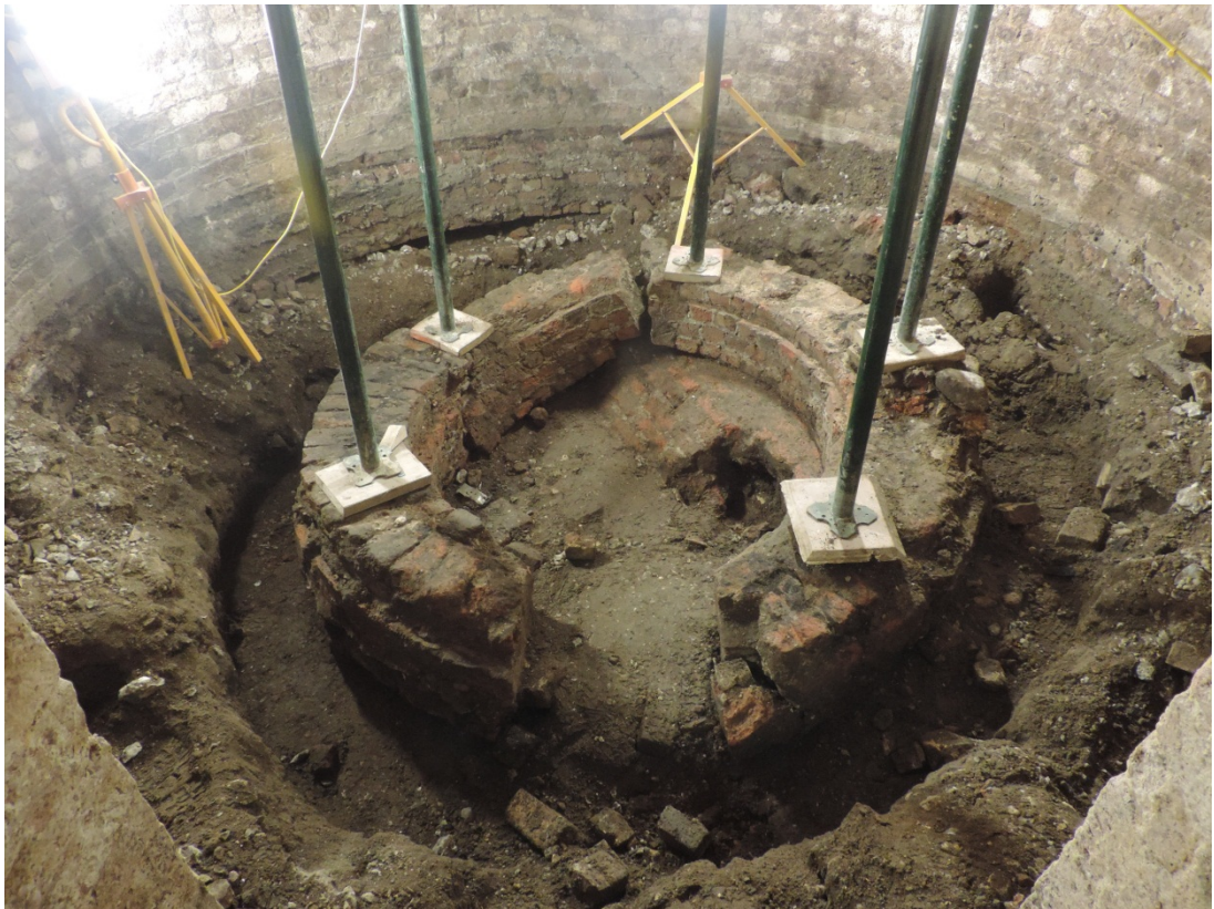
Fig 14 Circular brick feature exposed after the concrete floor of the Beehive was removed, looking south
