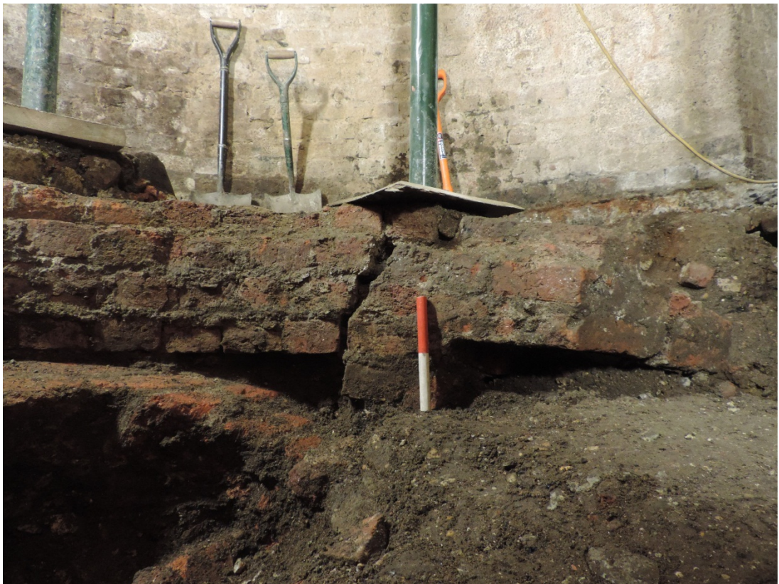
Fig 17 Northern break point of the collapse side of the wall, looking north-west
