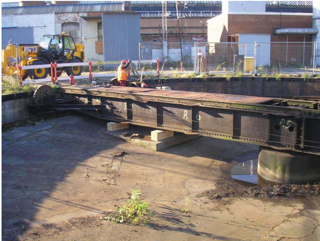
Plate 33. Turntable (right side) with deck and deck framework removed. The connecting cables of the locking bolt system seen here running along the side of the turntable were left in situ.
