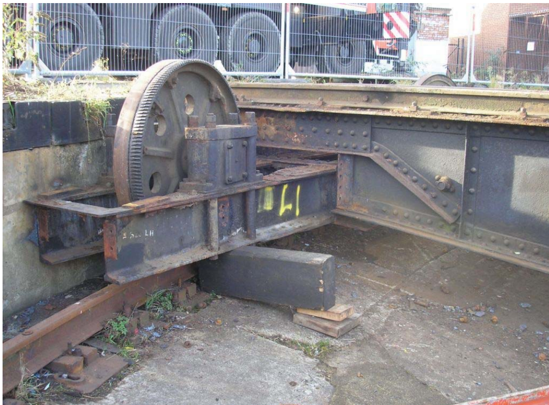
Plate 48. Manual drive wheel bogie secured with wooden blocks. The connecting bolts to the turntable main beam have been cut and the turntable itself jacked up slightly prior to lifting.
