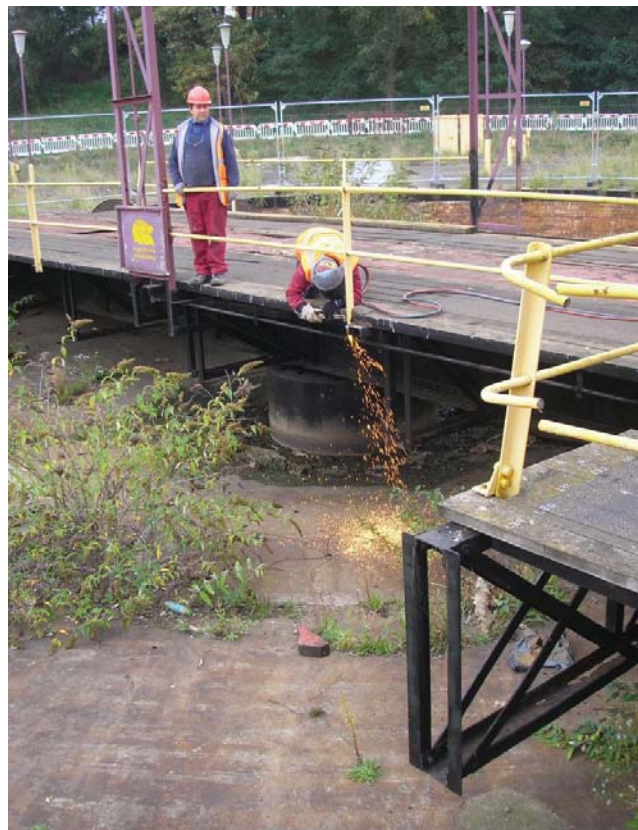
Plate 28. Handrail being removed. In foreground is truncated deck framework beneath electric operator's booth that once extended to support a deck enclosing the entire turntable pit.
