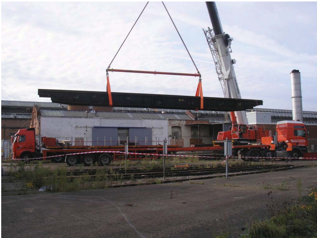
Plate 52. Turntable being lifted out of pit and positioned above a waiting lorry.
