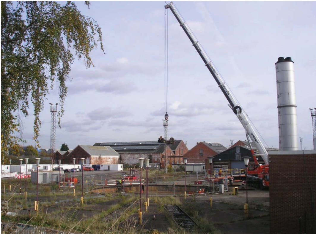
Plate 61. Turntable bogie being lifted out of turntable pit and onto a waiting lorry. Visible beyond are the brick gable ends of original 1905 Engine Shed buildings. The photograph is taken from approximately the same position as Plate 1.
