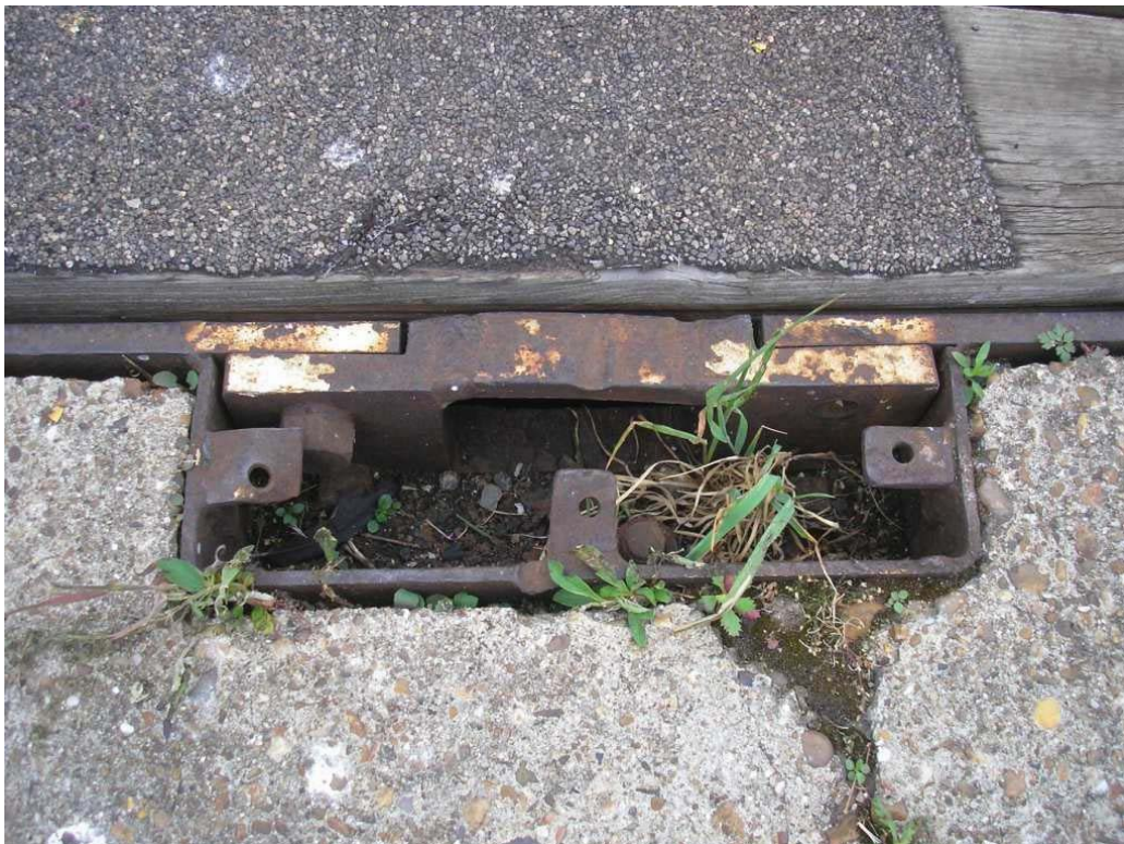
Plate 8. Locking plate for turntable with hole for locking bar from turntable found in between all tracks, here shown with cover plate missing.
