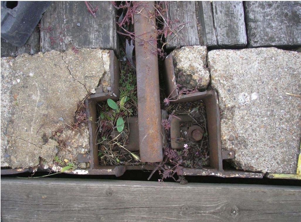
Plate 9. Junction of Engine Shed track and turntable deck at the bottom of the picture with covering metal plates removed, revealing metal side plates around rail retaining bracket.
