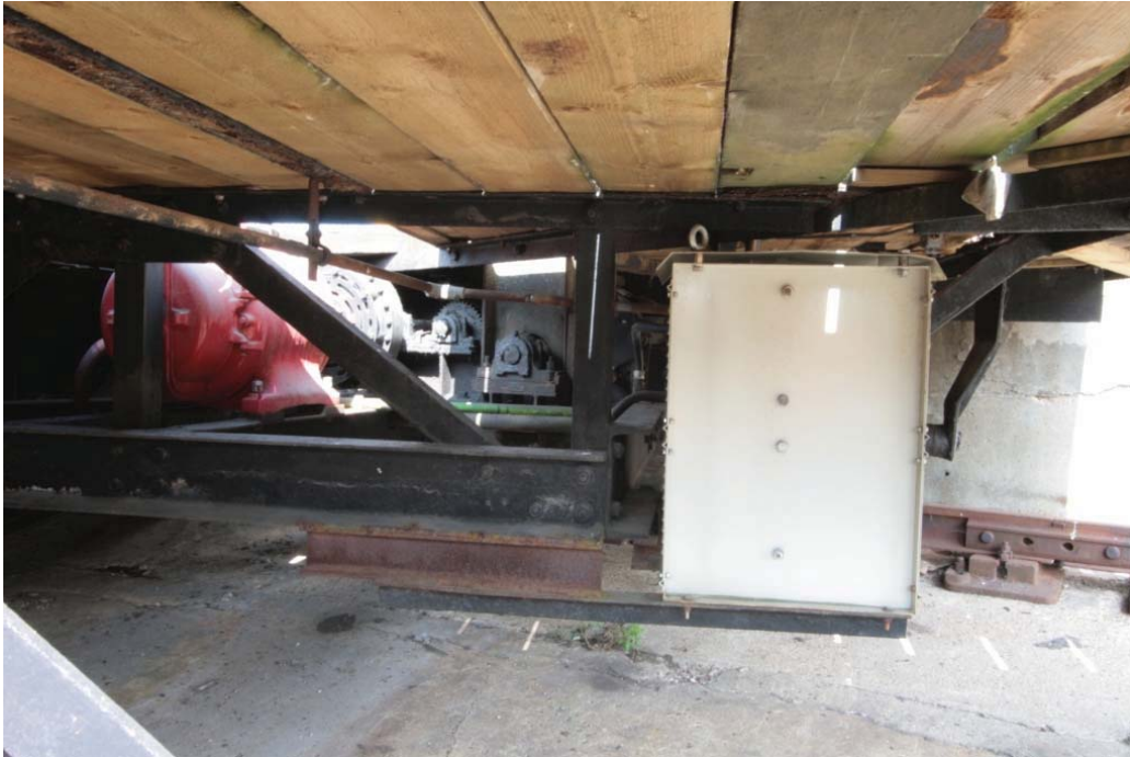
Plate 25. Electric drive motor on underside of turntable below operator's booth.
