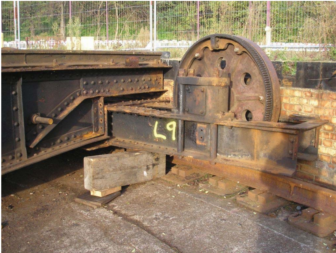
Plate 47. Electric drive wheel bogie secured with wooden blocks. The connecting bolts to the turntable main beam have been cut and the turntable itself jacked up slightly prior to lifting.
