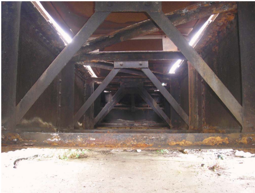
Plate 14. Underside of turntable between main beams looking toward outer edge, showing internal bracing covered by metal plates above fitted between the rails laid along the top of each main beam.
