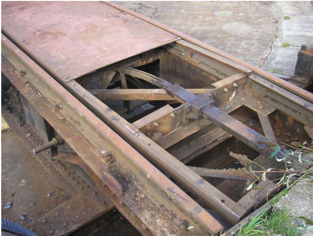
Plate 37. Locking bolt mechanism. The severed shaft on the left connected to the locking bolt lever which was left attached to the electric drive unit and removed.
