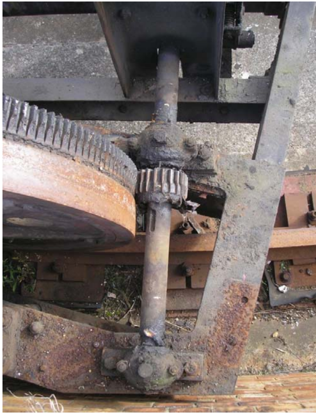
Plate 35. Detail of manual drive gearing, showing drive shaft, pinion and spur wheel.
