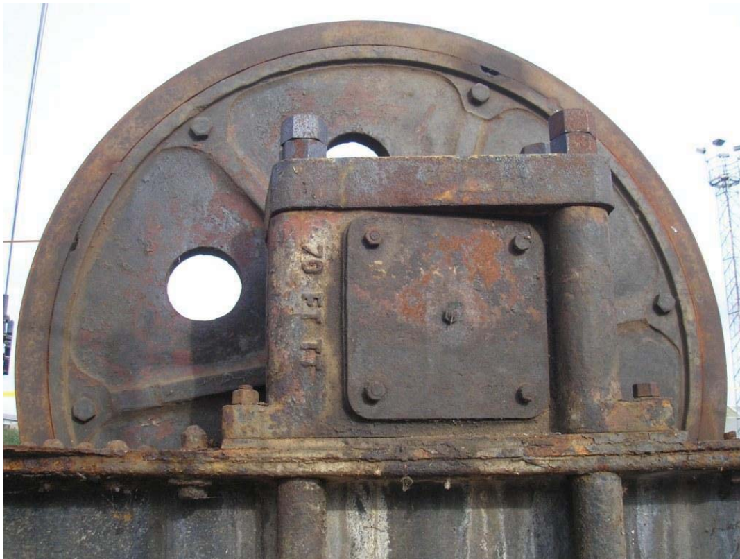
Plate 60. Outer face of manual drive wheel with '70FT TT' cast into axle bearing housing identifying the specific use of this component on this size of turntable.
