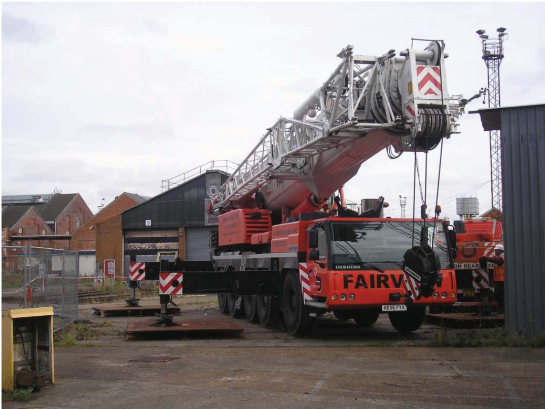
Plate 49. Mobile crane in position next to turntable pit, with steel pads beneath extended feet.
