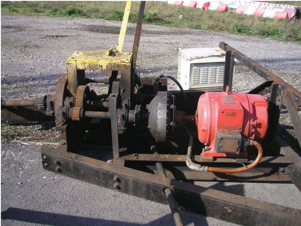
Plate 45. Electric drive unit with diagonal bracing beam and locking bolt shaft in foreground.
