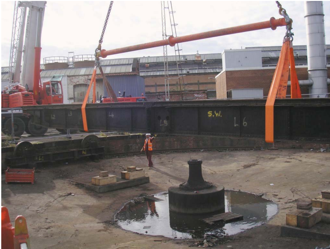
Plate 51. Turntable being lifted clear of central pivot and bogies and registering a weight of 22-tonnes on crane.
