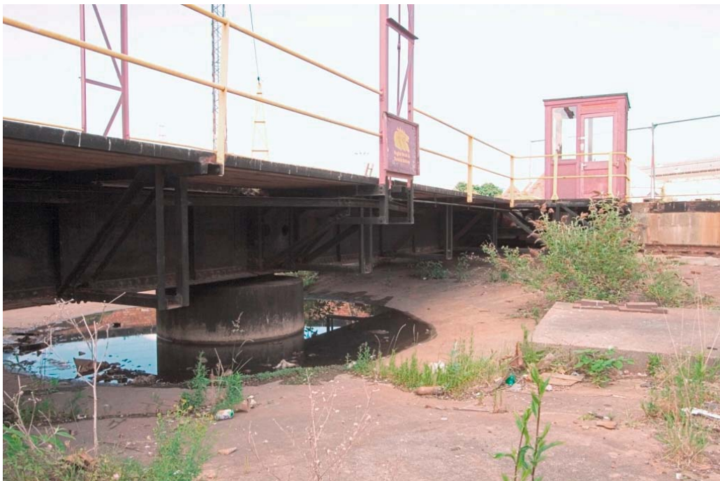
Plate 10. Side of turntable showing circular concrete pad for central pivot and horizontal section of concrete on right above sloping base of turntable pit.
