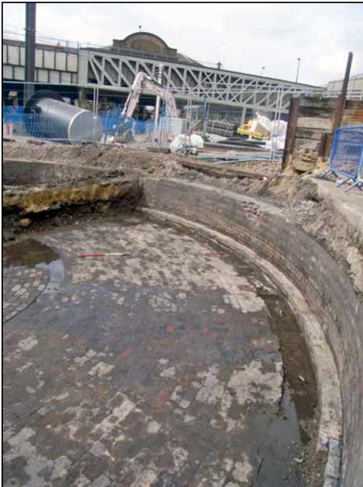
Plate 6: Guide rail gully [8523]
