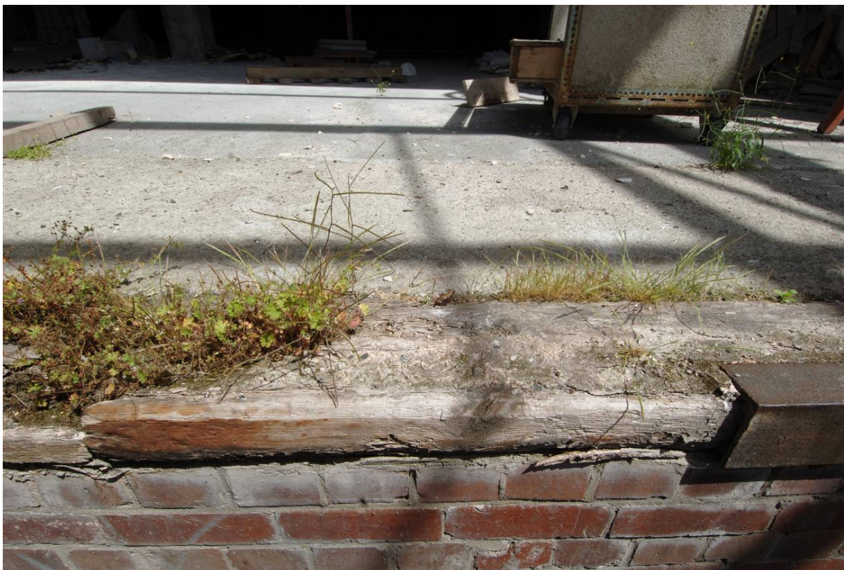
Fig 8 the timber and iron reinforcement along the edge of the southern platform, looking north
