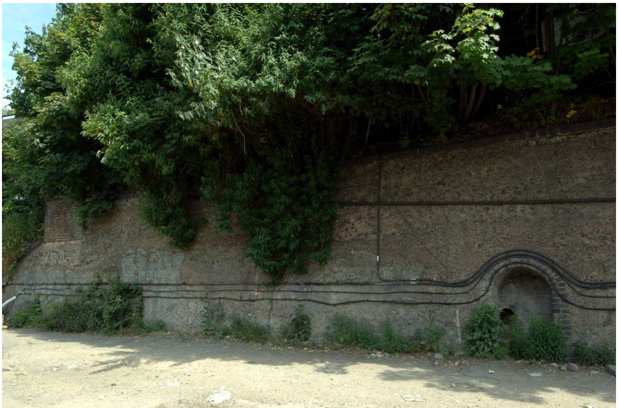
Fig 14 the 19th century retaining wall to the east of the building, looking north-west
