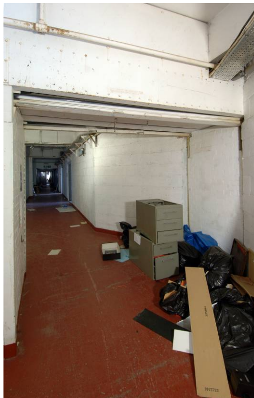
Fig 12 the fire door in the 1st floor corridor of the building, looking east
