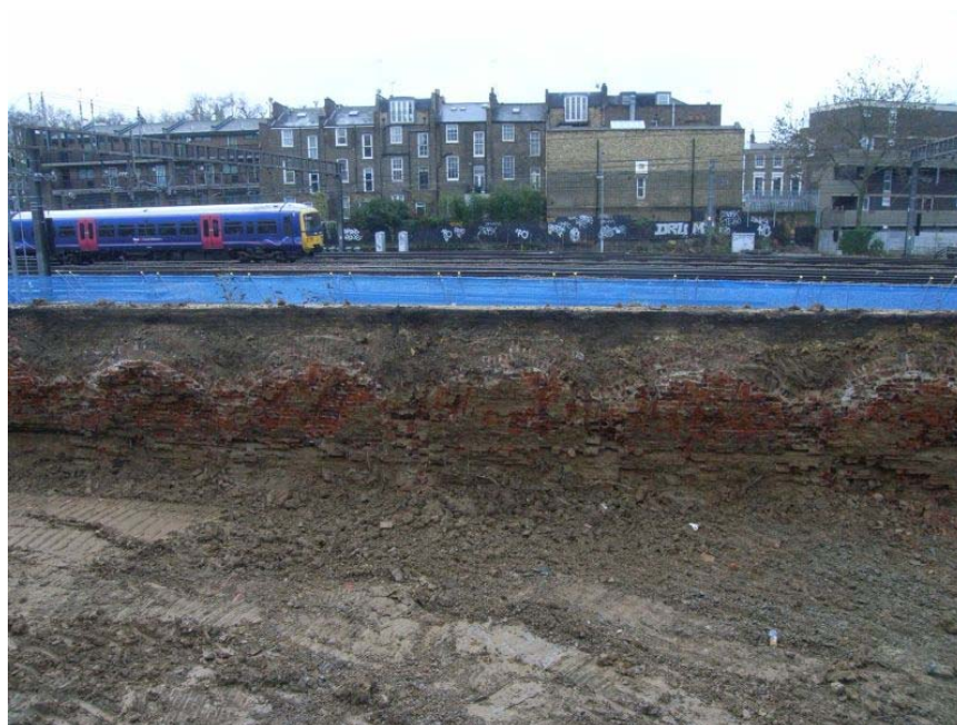
Plate 11: Arched brick structures 7025 along the southern side of the site, looking south
