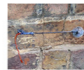
Vibrating Wire Crackmeter:
