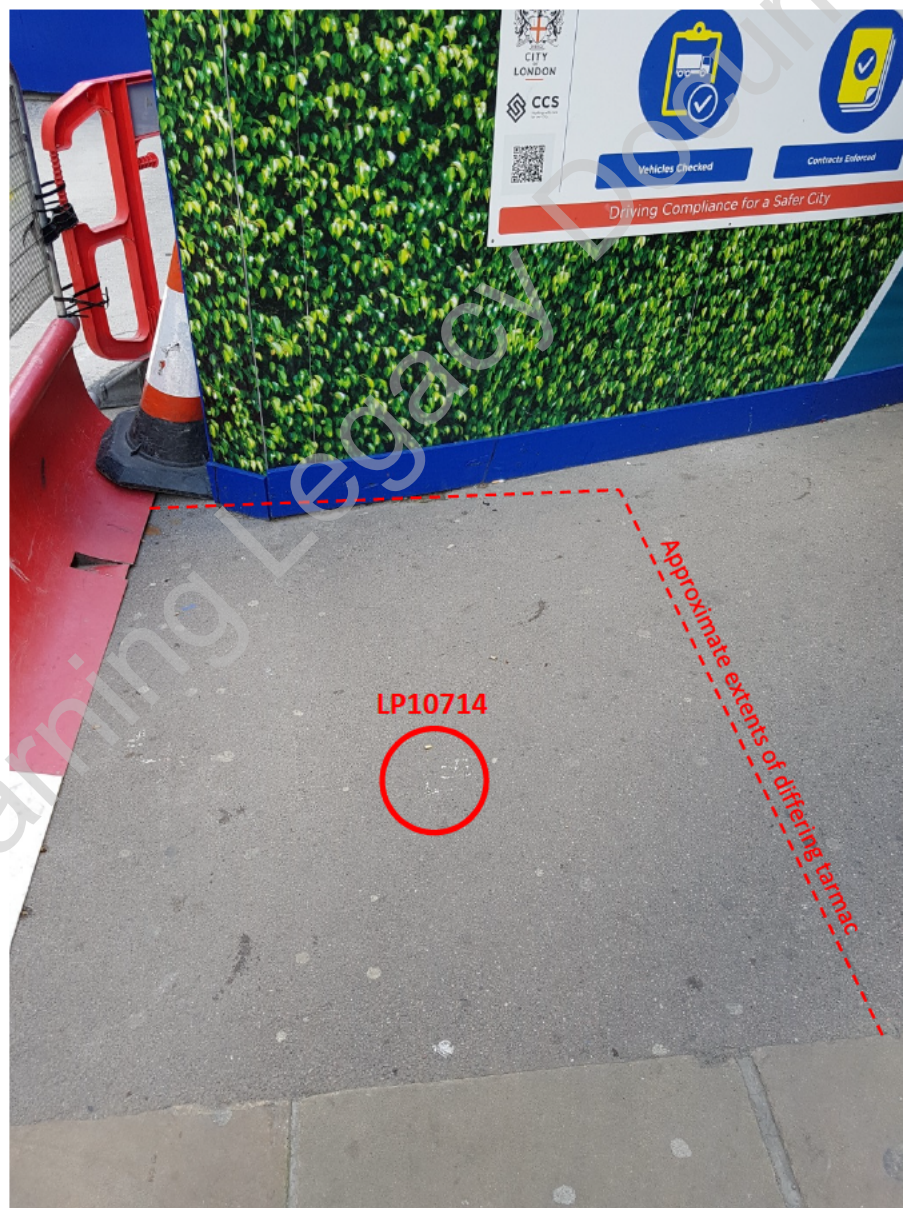
Figure 3- LP10714 Located on Unstable Pavement
