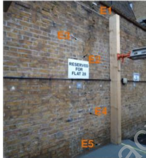
Blind Begger Crackmeter Locations
